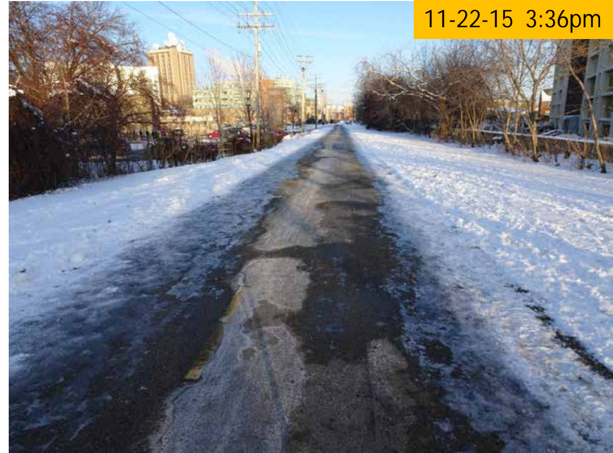
Section of path with BRINE PRE-TREAT (Corrosive residue emerging)
