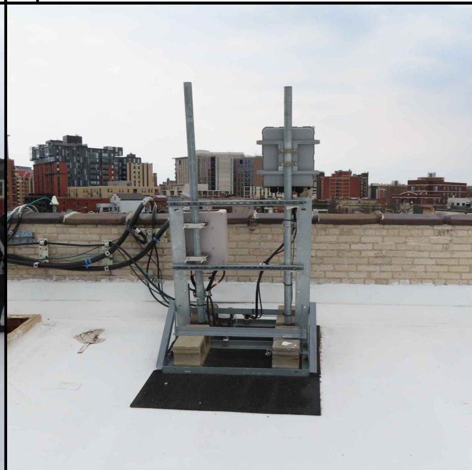
E EXISTING EQUIPMENT SLED MOUNT
