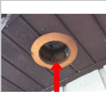
- Light fixtures in soffit are falling out or severely rusted. Appear to not work. Recommend repair
