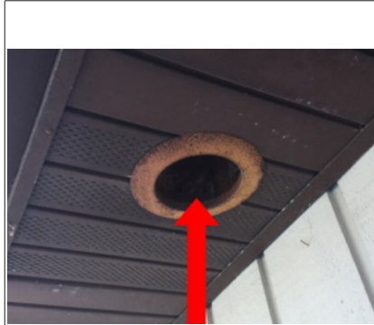
- Light fixtures in soffit are falling out or severely rusted. Appear to not work. Recommend repair
