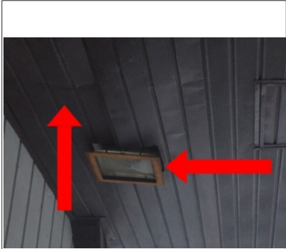
- Soffit has some damaged panels under canopy Recommend repair - Light fixtures in soffit are falling out or severely rusted. Appear to not work. Recommend repair
