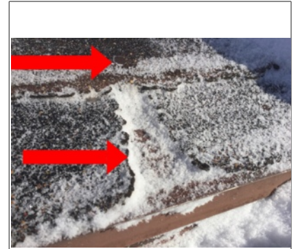
Shingles have broken corners, missing granulars and cracking. Recommend replacing soon
