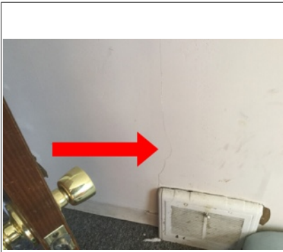
Crack in wall.
