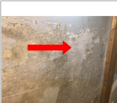
- Foundation has signs of Efflorescence. Recommend keeping water away from foundation wall on exterior.
