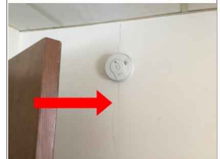
Crack in wall
