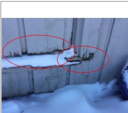
- Siding had some damage under north side door and at end of beam at west end of gable , recommend repairing/replacing damaged sections
