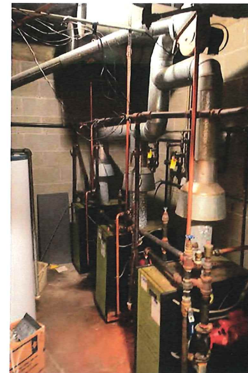
Mechanical room within original building
