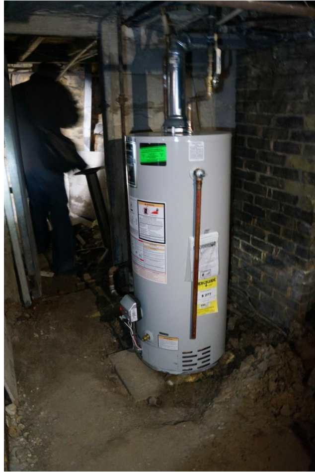
2. Basement – Water Heater
