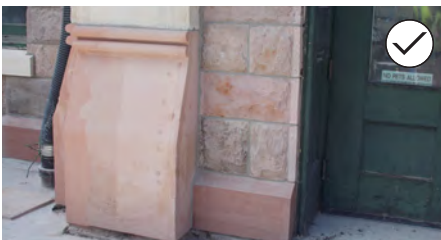
30. If necessary, repair a foundation wall using new material that is similar in character to the original. The foundation illustrated in the top image was patched with a consolidant that was tinted to match the existing pink sandstone, as illustrated below.
