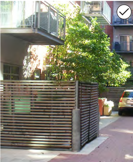
123. Screen ground-mounted mechanical equipment.
