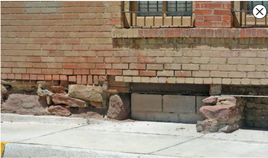
28. Do not allow an original foundation to fall into disrepair.
