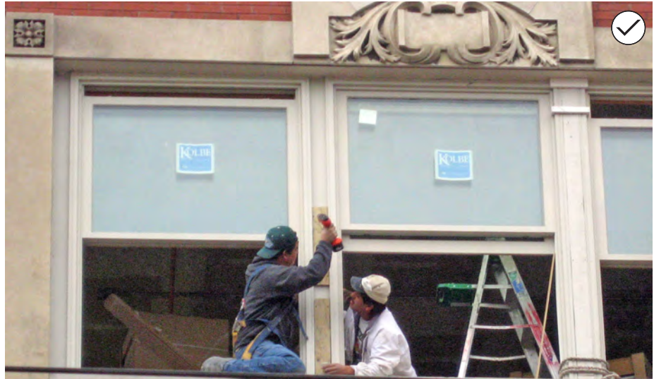
21. When replacement of an original window is necessary, match the replacement design to the original.
