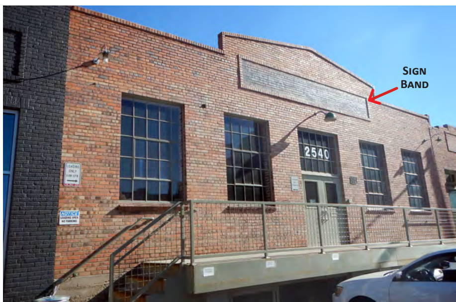
133. This building has an original sign band centered over the front door which would be a good signage location for a future user.
