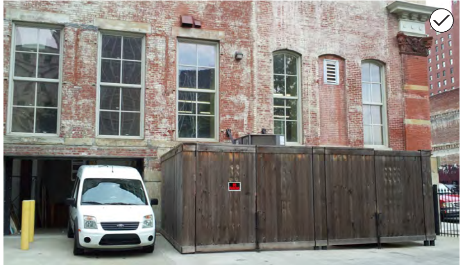
124. Locate service areas and ground-mounted mechanical equipment to the side or rear of buildings.
