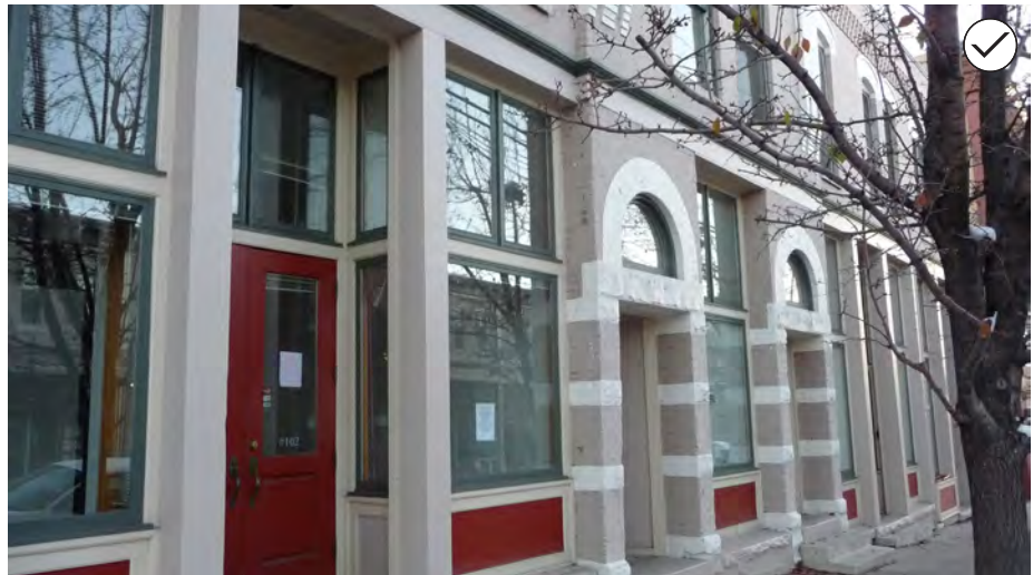
46. If necessary, replace windows with thermal pane glass, similar in appearance to the original, on a historic storefront.
