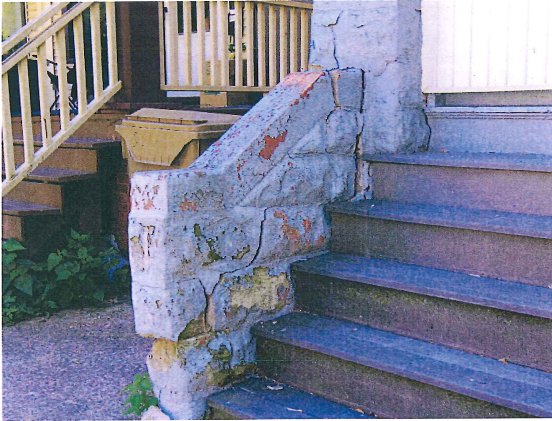
Severely damaged handrail – to be replaced
