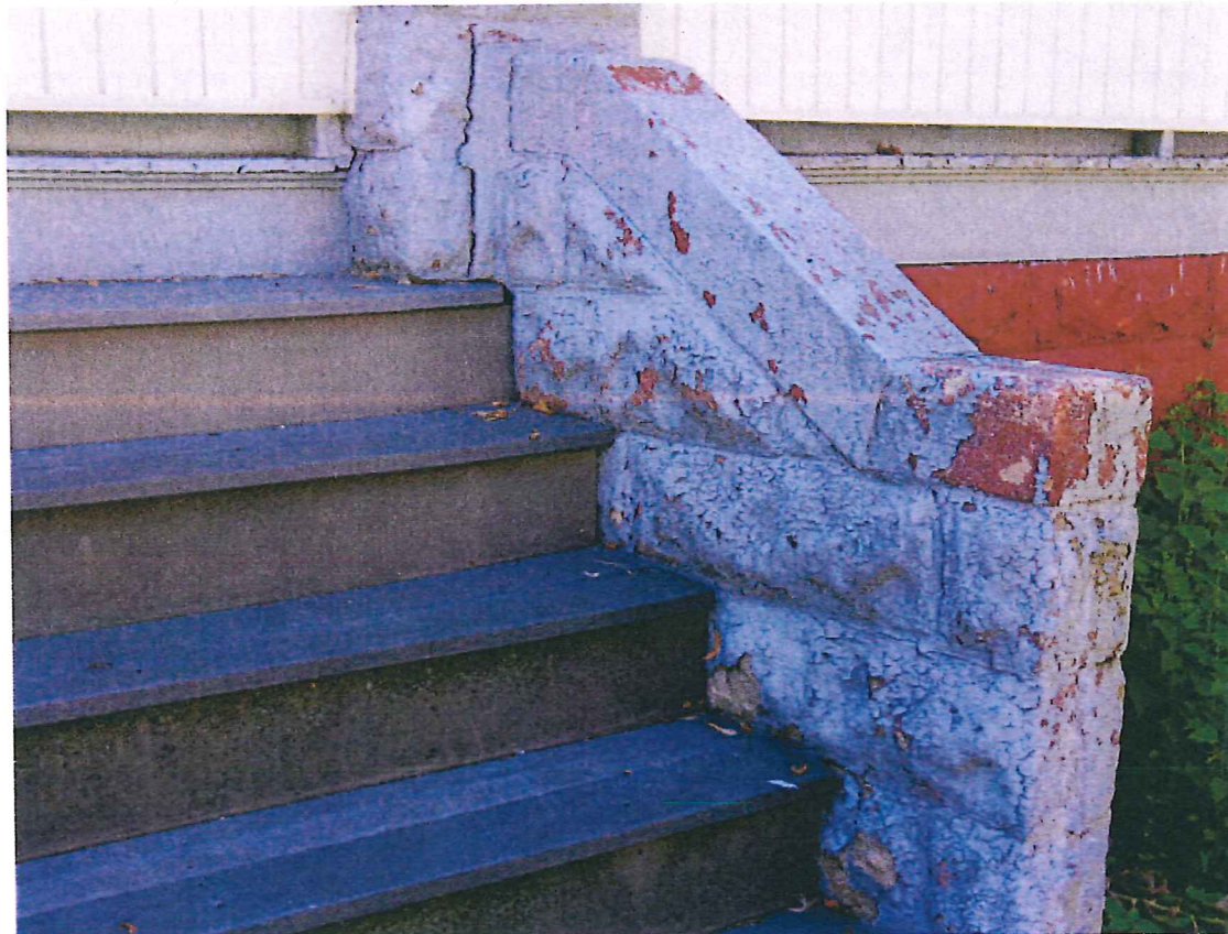
Damaged handrail – to be replaced
