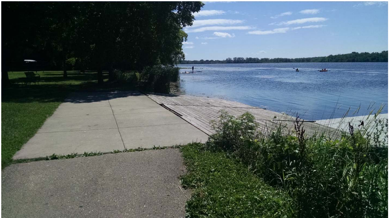
The wooden pier has rotted decking and is a potential hazard. The concrete abutment is in good condition and will remain in place. A new, permanent dock structure will be built off the existing abutment. The floating dock attached to the wooden pier will be relocated to the smaller concrete abutment on-site.
