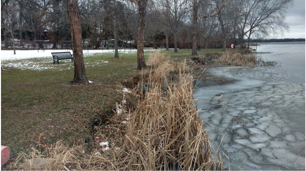
Although the shoreline appears stabilized from a distance, the existing vegetation is not adequately holding the bank.
