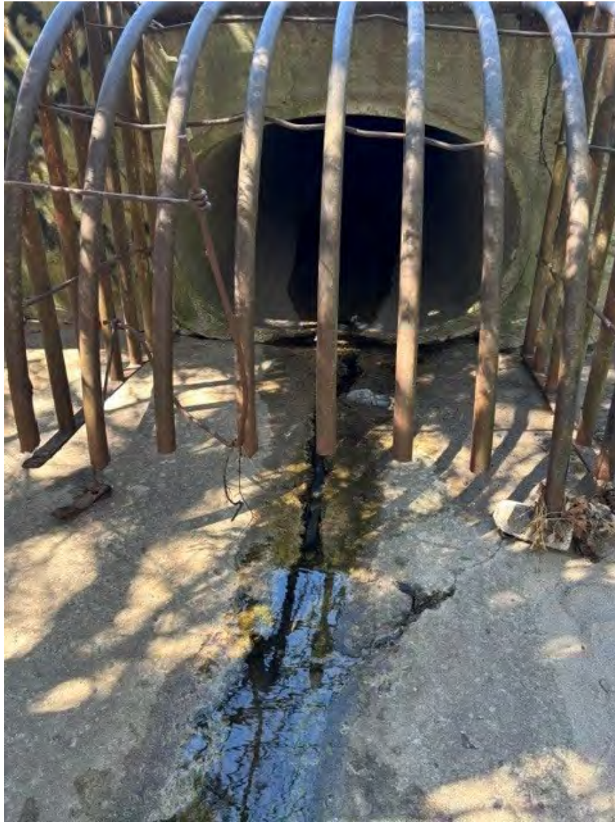
West End Headwall – Needs new pipe gate & under-pipe repair
