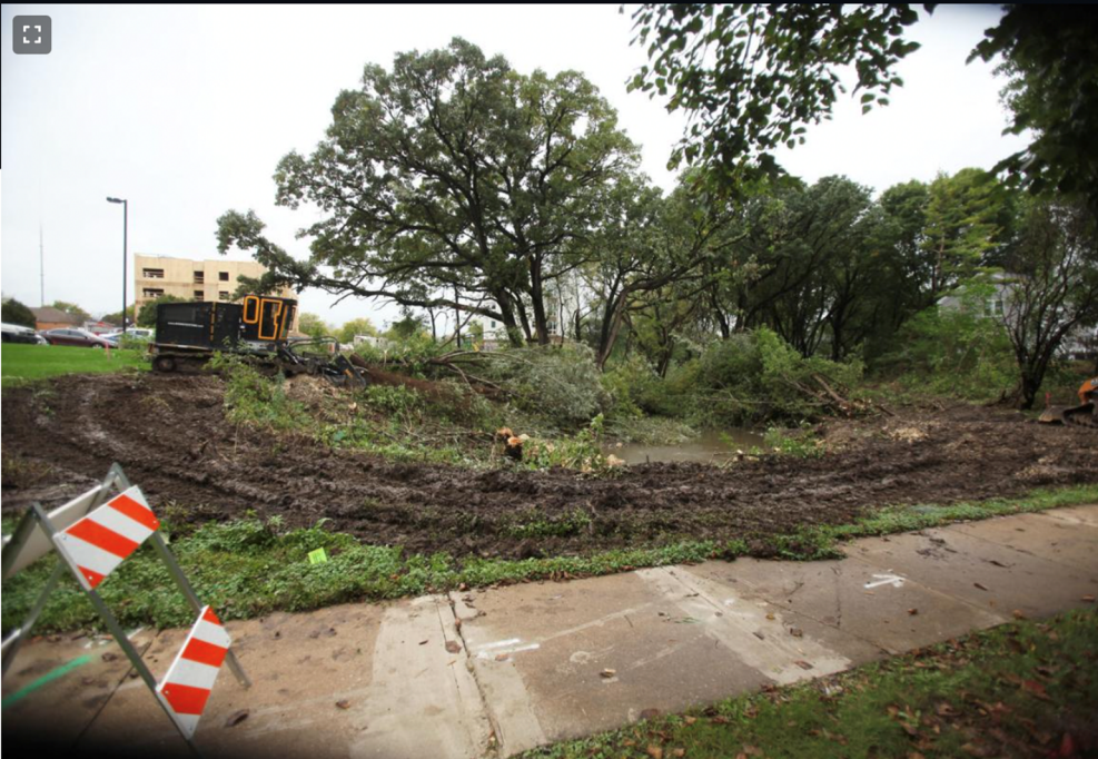
More than 200 trees were removed from a Far West Side green space at the beginning of October. The cuts were made as part of a restoration project.
