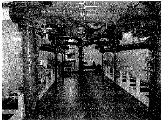
Photos of Middleton, WI Plant toured by Utility Staff
