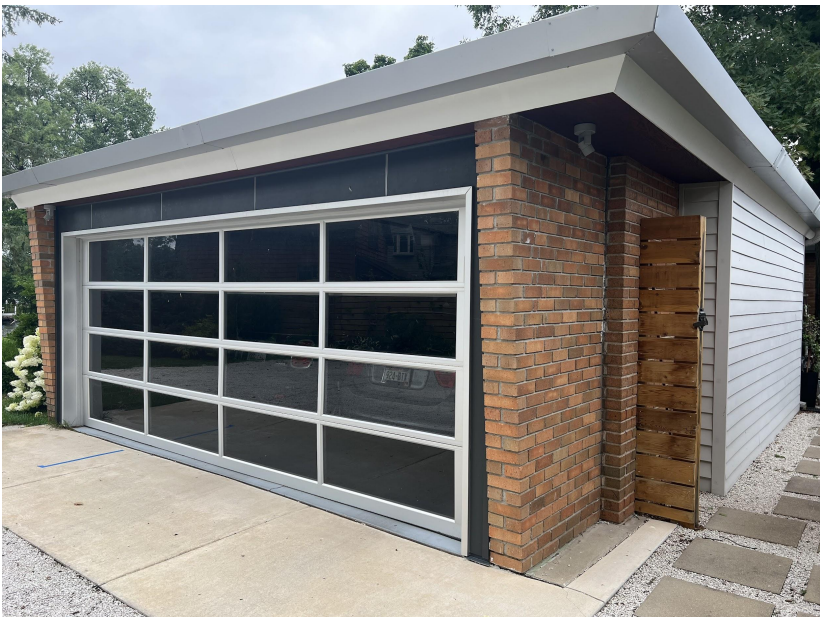
Close-up view of the existing garage which will be demolished and rebuilt as a part of the overall addition project.
