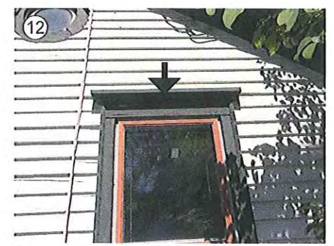
12 Repair/replace cracked trim
