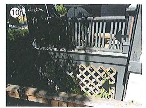
10 Replace deteriorated railing; replace lattice
