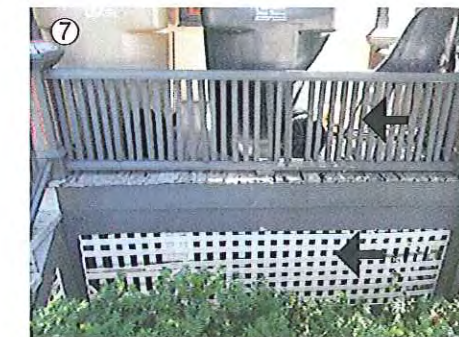
7 Replace deteriorated railing; replace lattice
