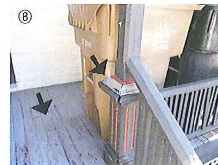
8 Repair/replace column trim; replace all floorboards
