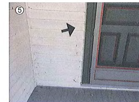
5 Replace cracked siding
