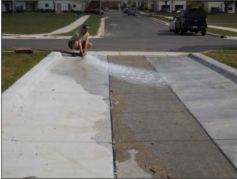
Photo 2: Eric Hopper of the Water Utility water flooding with a fire hose.
