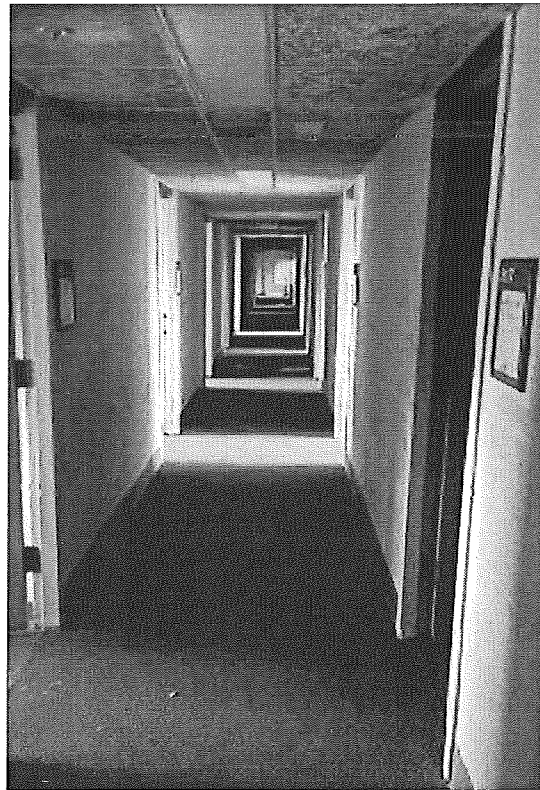
Figure 8: Fifth Floor Mold on Ceiling Tiles.
