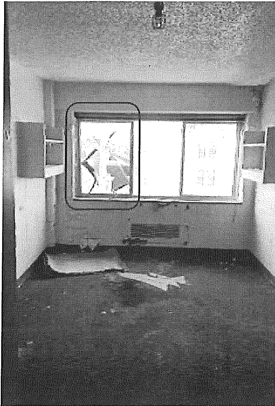
Figure 9: Fourth Floor Broken Window.
