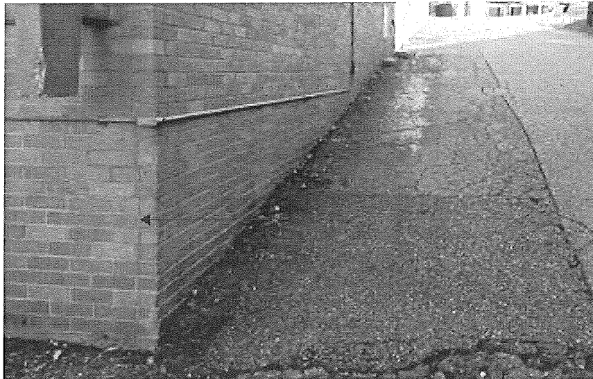
Figure 5: Northwest Corner Brick Veneer Cracking.
