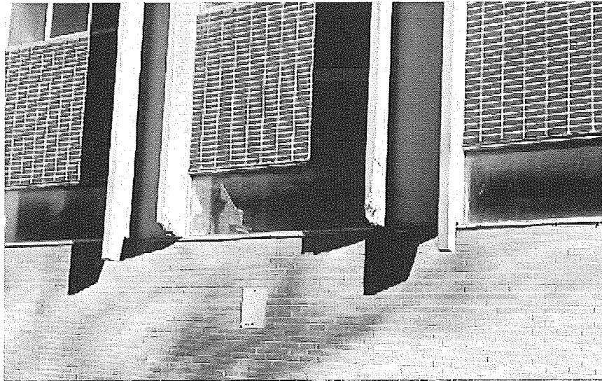
Figure 3: West Elevation Broken Precast Cladding.
