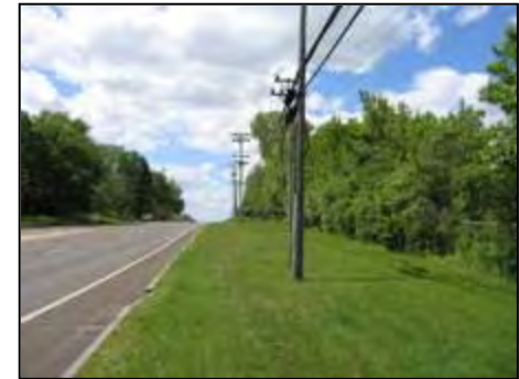
FIGURE 2.33 Utility Lines along University Avenue
