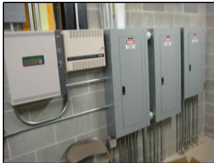
EXISTING AC ELECTRIC PANELS IN UTILITY ROOM
