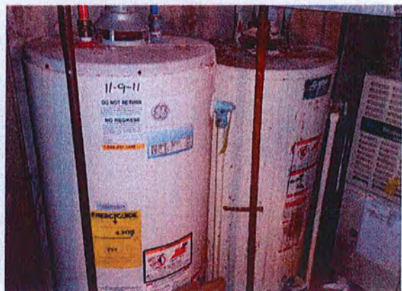
Water heaters with >5 years life remaining
