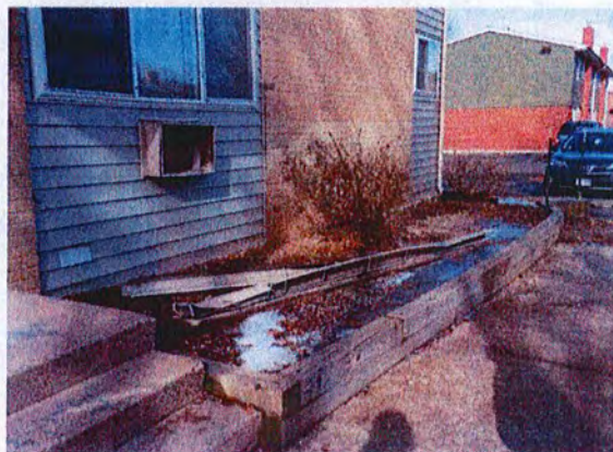
Exterior landscaping beams (6x6)
