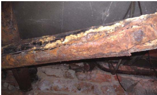
Deteriorated sanitary pipe
