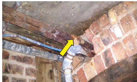
Deteriorated gas pipe
