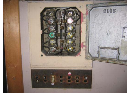
Electrical fuse panel on 1 st floor.
