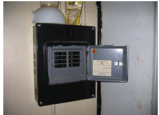
Electrical panel on 2 nd floor.
