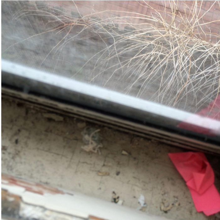
Rear bedroom (Southeast corner), Broken and missing glass, dry rot to bottom rail lower sash missing glass in storm.
