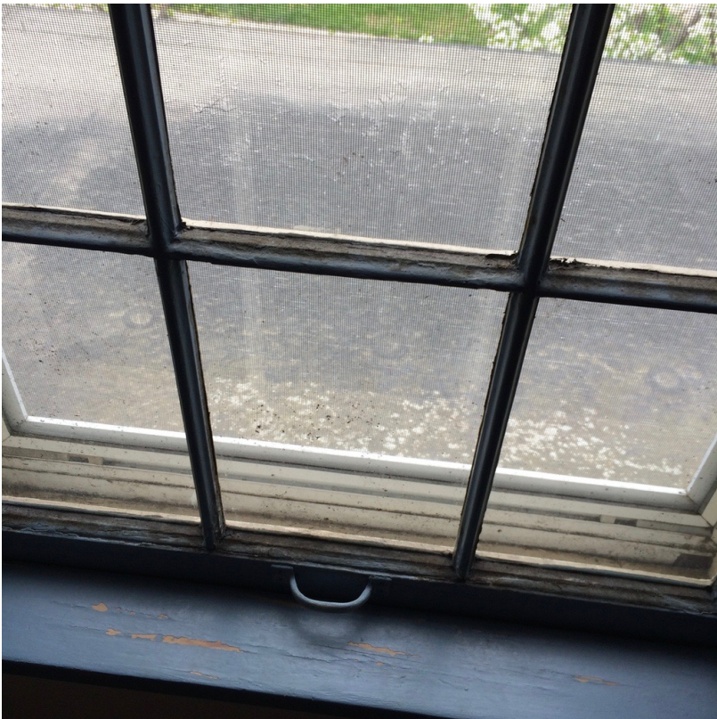
Front bedroom (Northeast corner) excessive mold dry rot and sill damage
