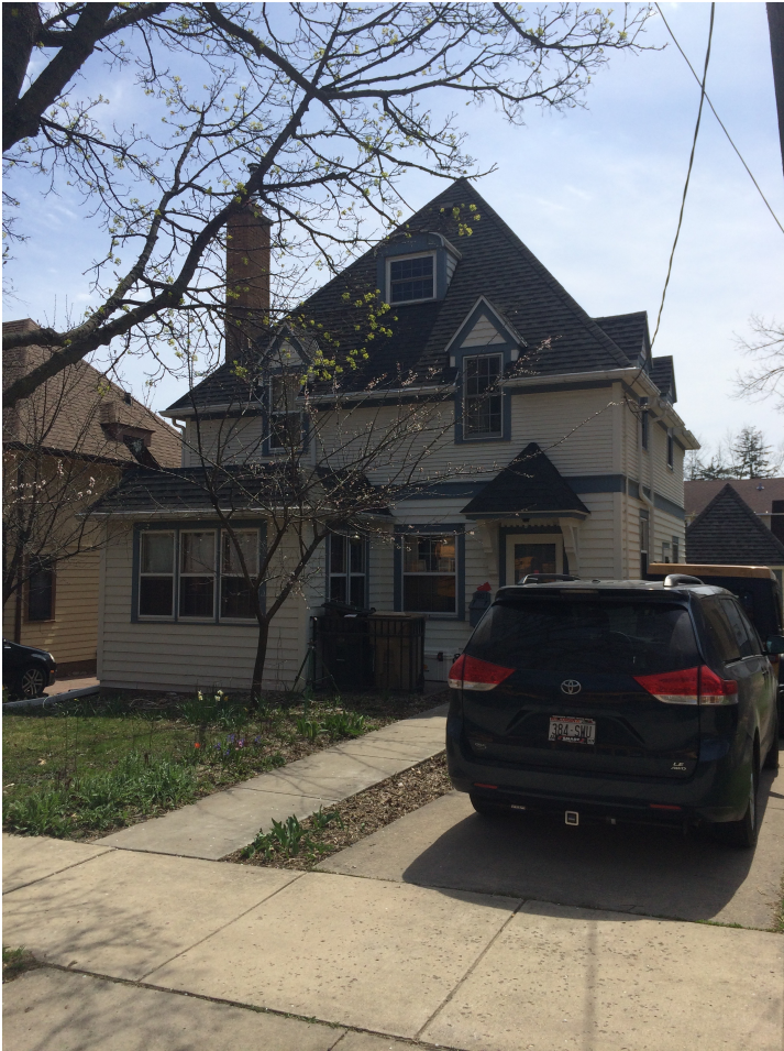
Front exterior Upper windows on right side (Northwest) are new Marvin inserts
