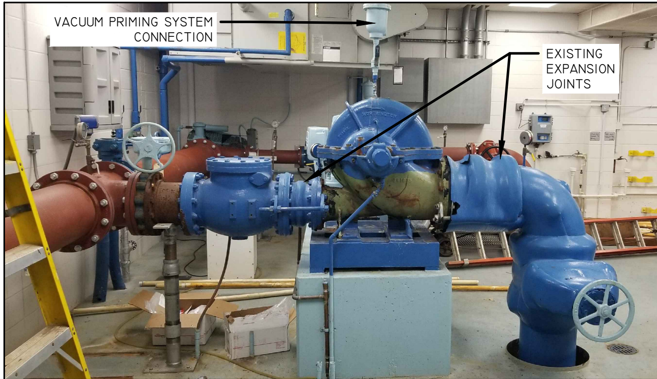
BOOSTER PUMP #2 SIDE VIEW / PUMP SIDE
