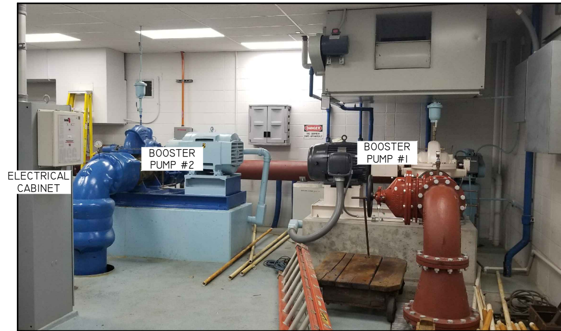
VIEW OF PUMPS FROM DEEP WELL
