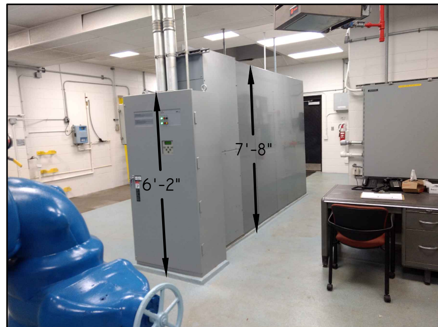
ELECTRICAL CABINETS TOWARD DEEP WELL (OBSCURED)
