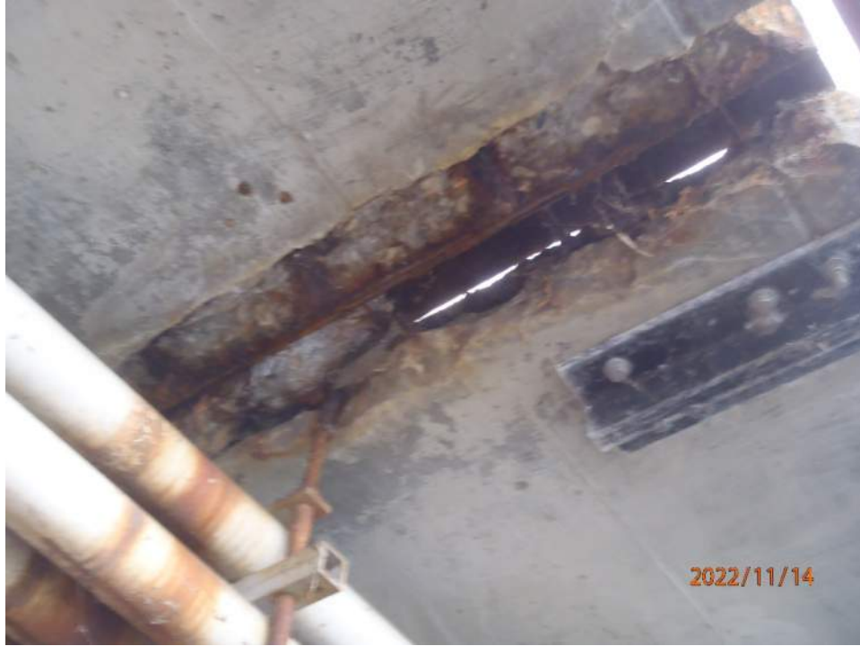
Photo 1: Typical sidewalk expansion joint spall
