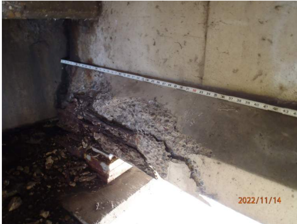
Photo 2: Typical girder end spall
