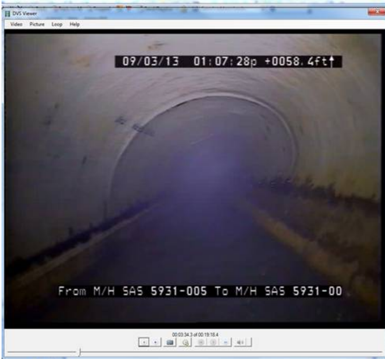
24" liner is in process of collapsing
