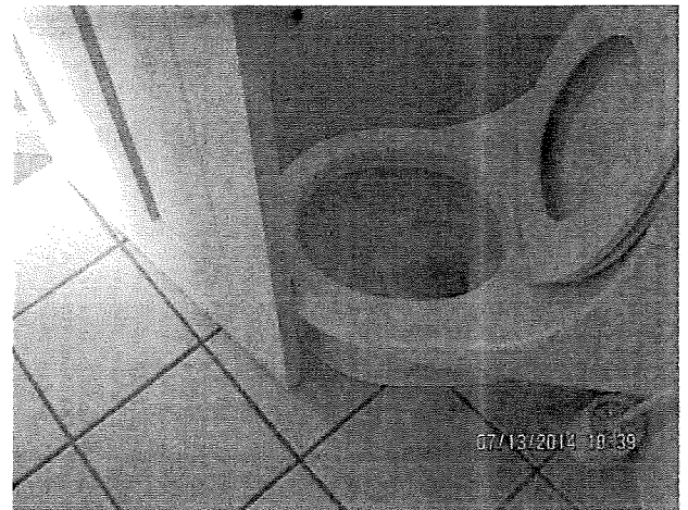
315 S. Mills St. CONDITION EXAMPLES MAIN BATHROOM
