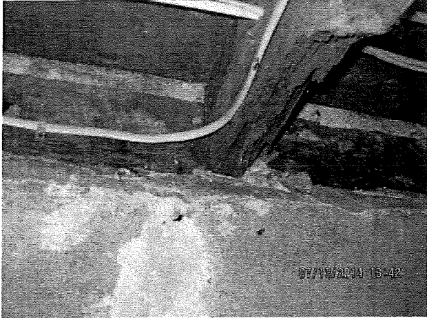
315 S. Mills St. CONDITION EXAMPLES FLOOR JOIST ROT AT FOUNDATION WALL
