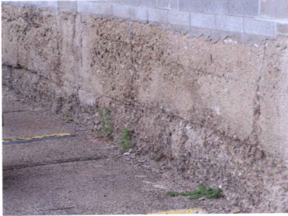
644 Mifflin Street Cracked Foundations May 9, 2005
