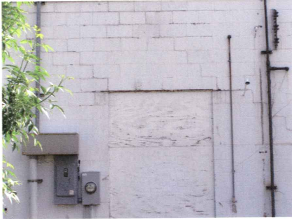
202 South Thorton Blocks Displaced Wall Cracked Wall Bolt May 28, 2005
