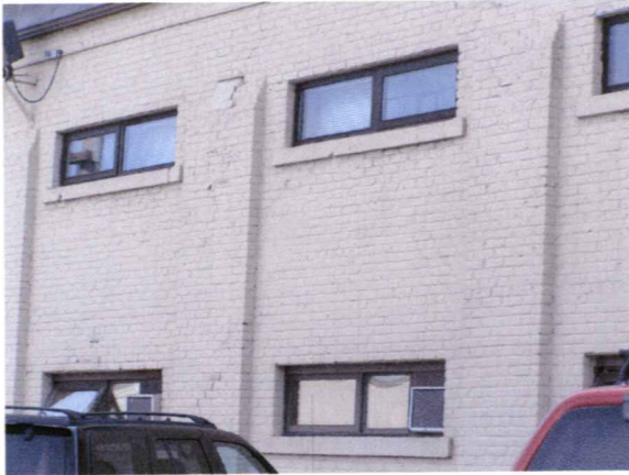
1011 – 1015 Main Street Wall Cracks May 25, 2005
