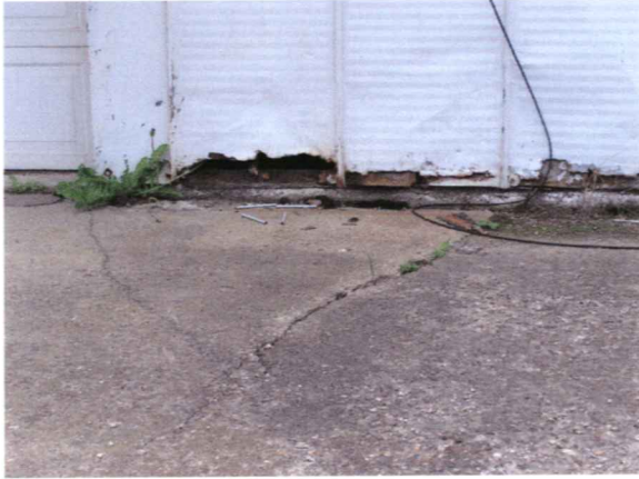
1415 Dayton Street Wall Rusted Away Loading Deck Cracked May 28, 2005
