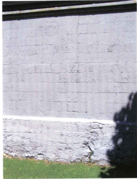
222 South Baldwin Cracked Wall Cracked Foundation May 28, 2005
