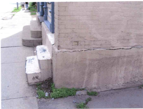
912 Williamson Steps Protruding Into Sidewalk No Handrail Steps Are Steep Foundation Parged & Loose May 21, 2005
