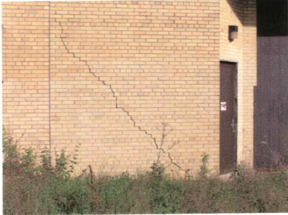
1043 East Wilson Street Cracked Wall May 26, 2005
