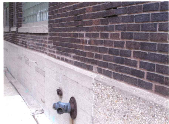
849 East Washington Avenue Pedestrian Impediment Deteriorated Foundation Deteriorated Mortar May 17, 2005
