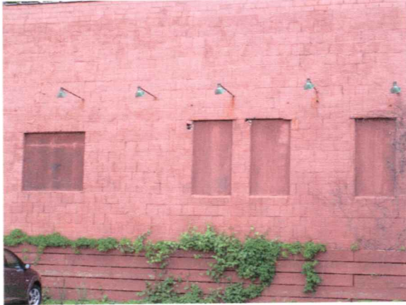
1001 East Washington Avenue Windows Boarded Up Wall Cracks Holes in Blocks May 25, 2005
