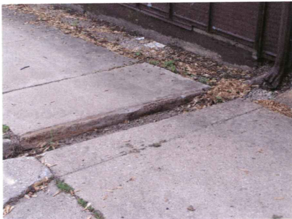
1354 East Mifflin Street Gap In Sidewalk Cover Plate Missing Dented Downspout May 28, 2005
