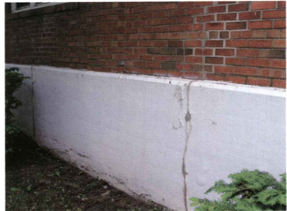
1450 Main Street Cracked Wall Cracked Foundation May 28, 2005
