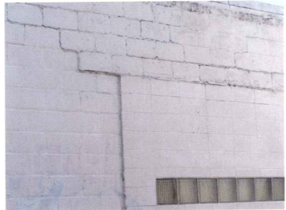
940 Williamson Cracked Wall Blocked-up Door May 21, 2005
