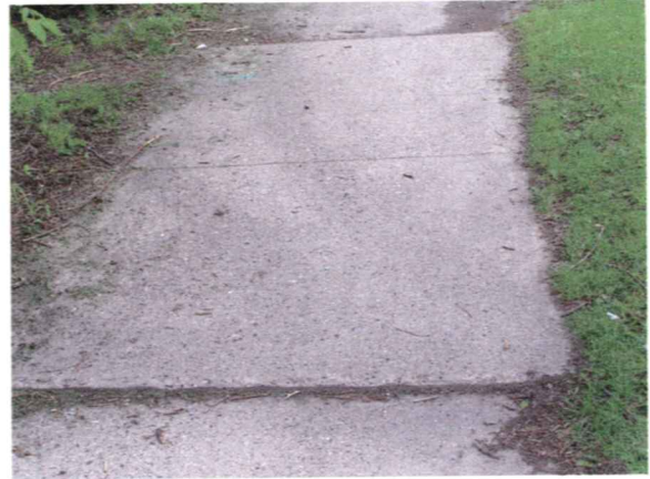
607 East Mifflin Street Uneven Sidewalks May 17, 2005
