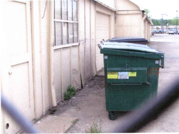
815 East Washington Avenue Broken Windows Dented & Loose Wall Panels Inadequate Outdoor Storage
