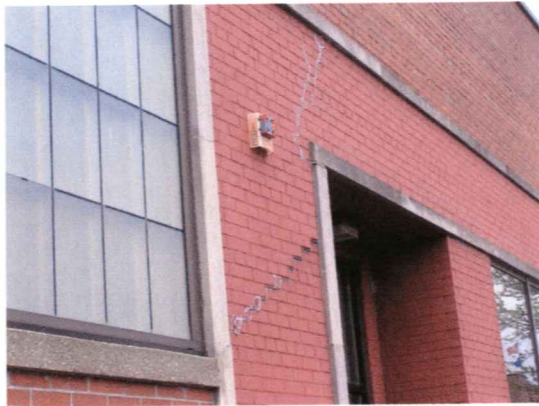
600 Williamson Street Cracked Wall May 9, 2005
