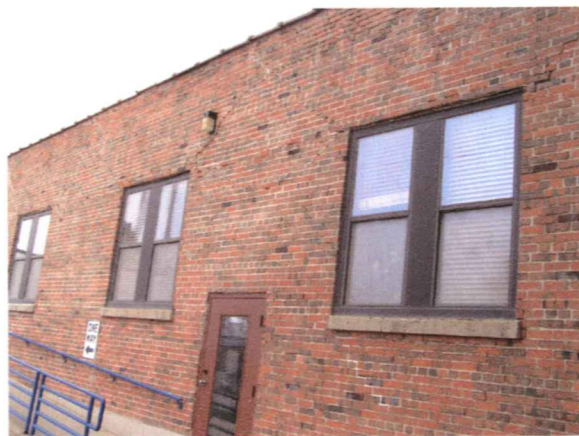
849 East Washington Avenue Multiple Wall Cracks May 17, 2005
