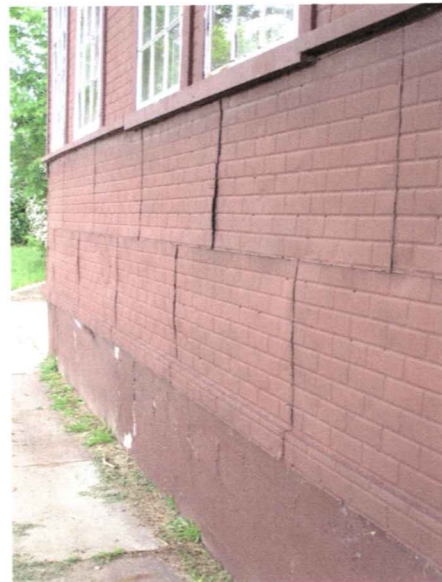
1354 East Mifflin Street Cracked Foundation Loose Siding Deteriorated Window Frame May 28, 2005
