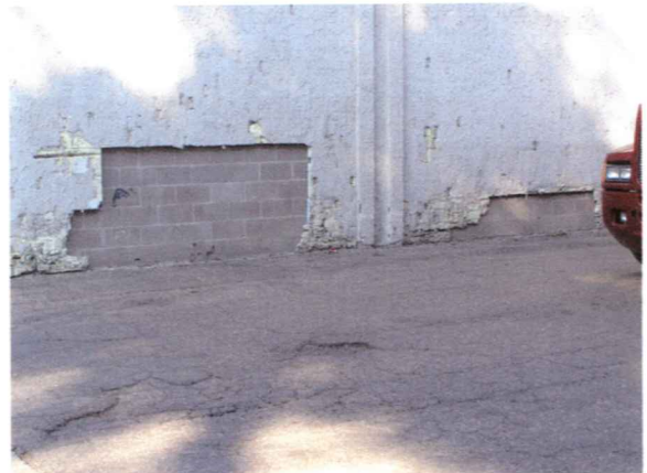
1025 East Mifflin Street Stucco Missing May 24, 2005
