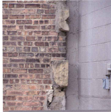
115 South Blount Street Deteriorated Brick May 9, 2005
