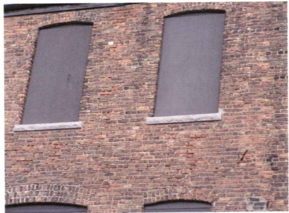
115 South Blount Street Boarded-up Windows May 9, 2005
