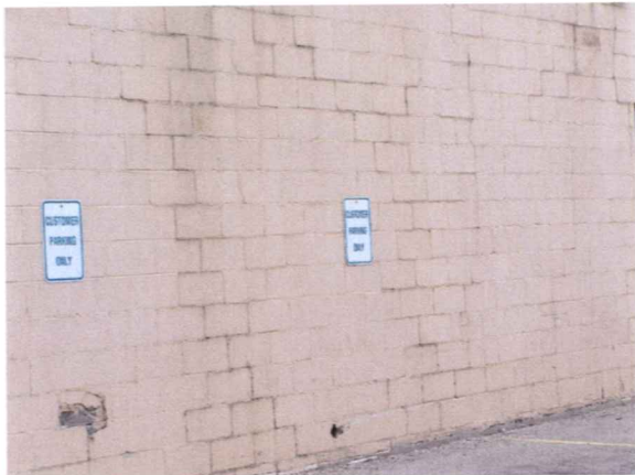
939 Washington Wall Cracks May 24, 2005
