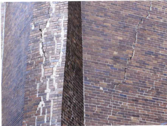
619 East Washington Avenue Wall Cracks May 9, 2005
