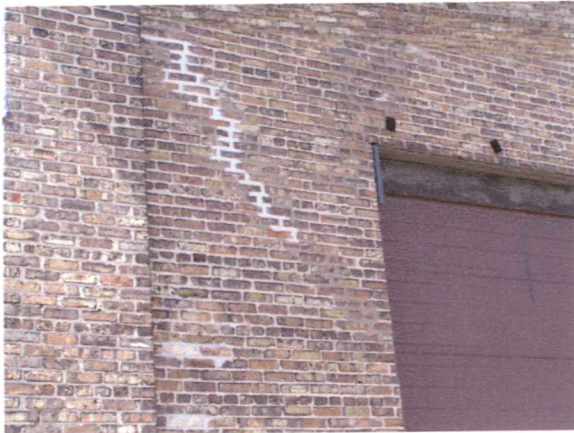
1245 East Washington Avenue Cracked Wall May 28, 2005
