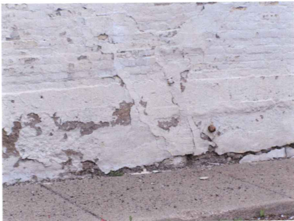
627 Mifflin Street Foundation Cracked Foundation Bolt May 17, 2005
