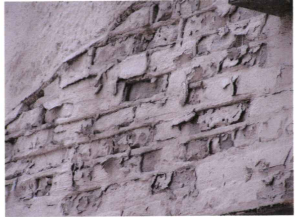
917 East Mifflin Deteriorated Brick May 24, 2005
