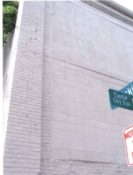
202 South Thorton Blocks Displaced Wall Cracked Wall Bolt May 28, 2005
