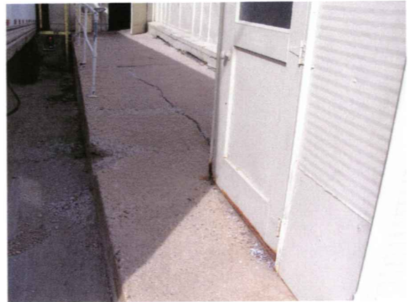
1011 Main Street Rusted Door Broken & Deteriorated Porch May 25, 2005
