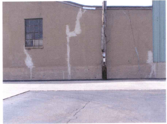
701 East Mifflin Cracked Wall Broken Window May 17, 2005
