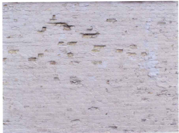
627 Mifflin Street Wall Cracks May 17, 2005
