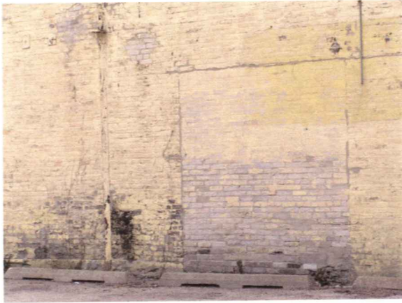
627 Mifflin Street Deteriorated Wall May 17, 2005
