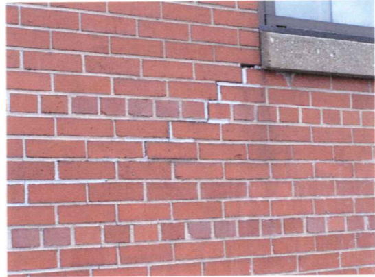
600 Williamson Street Cracked Wall May 9, 2005
