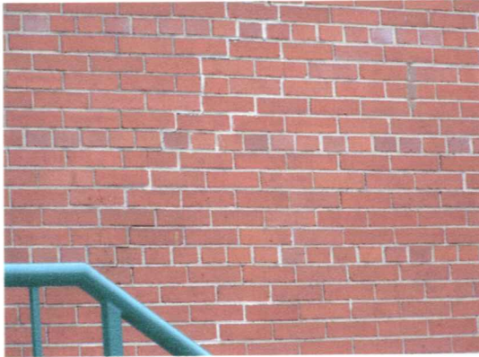
600 Williamson Street Cracked Wall May 9, 2005
