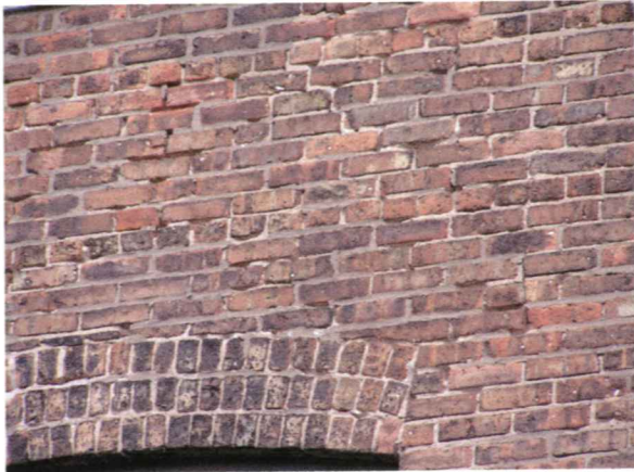
115 South Blount Street Deteriorated bricks May 9, 2005
