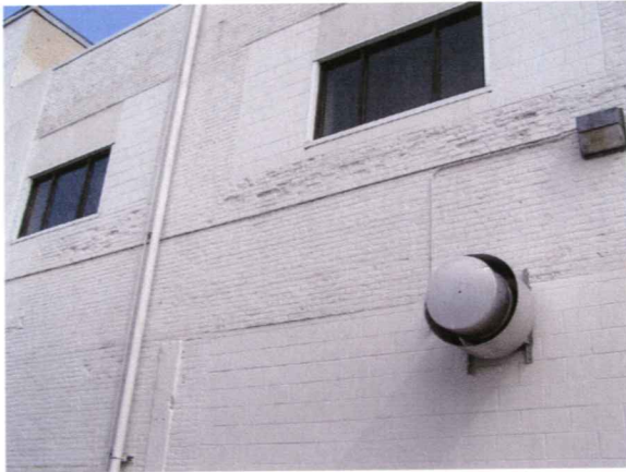
702 East Washington Deteriorated Brick Blocked Windows May 17, 2005
