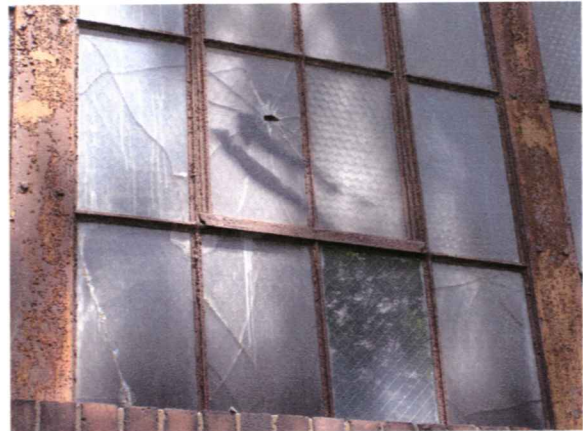
901 East Washington Rusted Frames Broken Glass May 24, 2005
