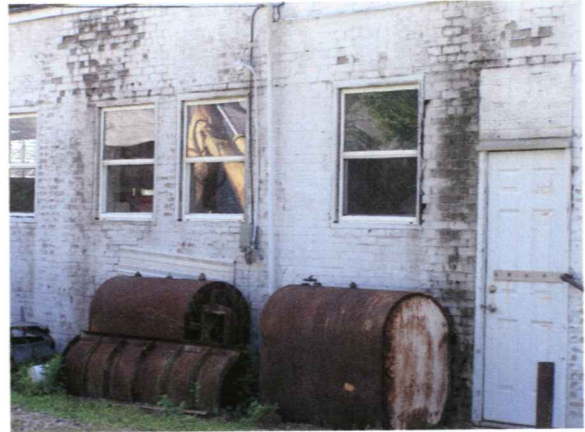
1200 East Washington Avenue Deteriorated Bricks Blocked- up Door Deteriorated Door May 28, 2005
