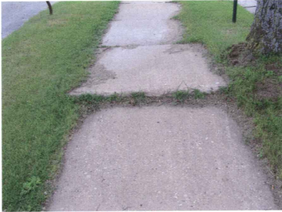
1451 East Washington Avenue Dangerous Sidewalk May 28, 2005
