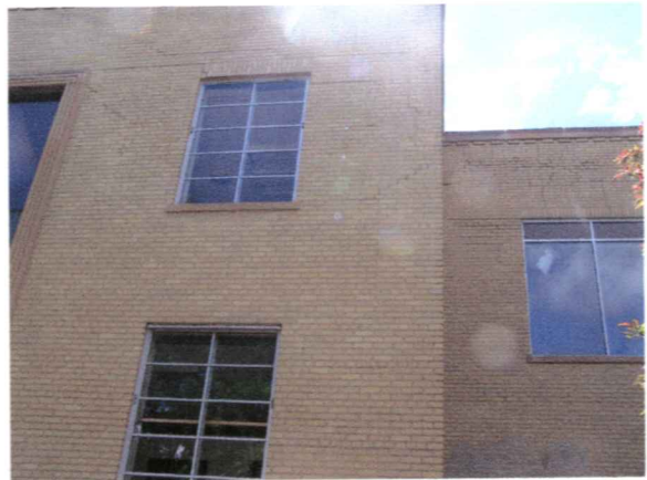
1450 East Main Street Cracked Wall May 28, 2005
