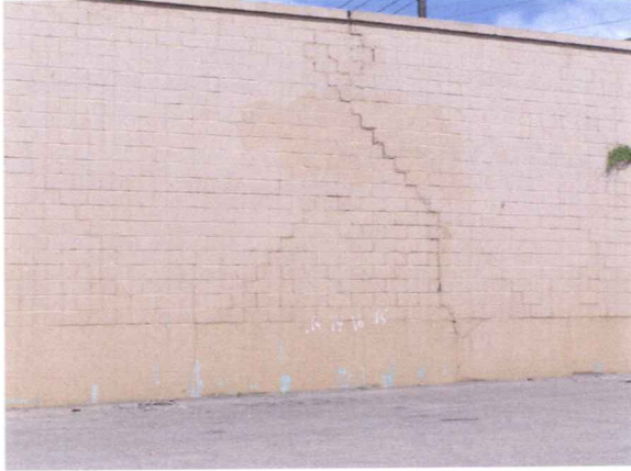
925 East Washington Wall Cracked May 24, 2005
