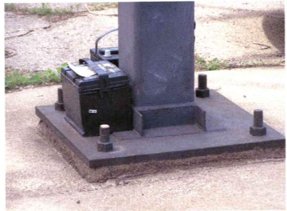
741 East Mifflin Batteries Stored Outdoors May 17, 2005
