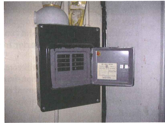
Electrical panel on 2 nd floor.
