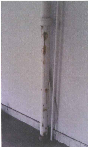
Leaking sanitary pipe
