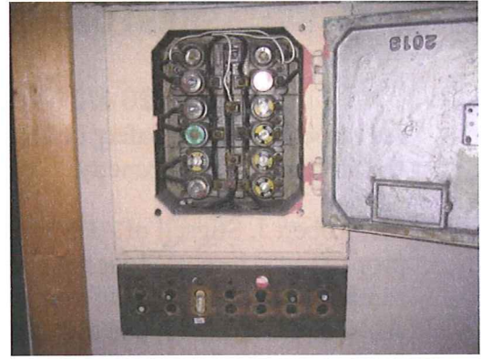
Electrical fuse panel on 1 st floor.
