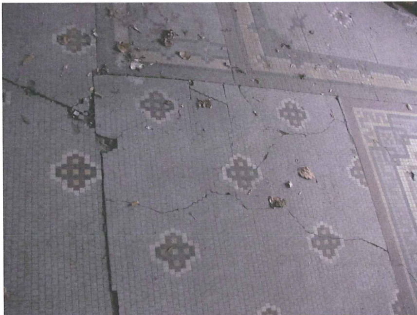
Figure 14. There is elaborate mosaic tile flooring at the first floor; the flooring has suffered extensive cracking and displacement.
