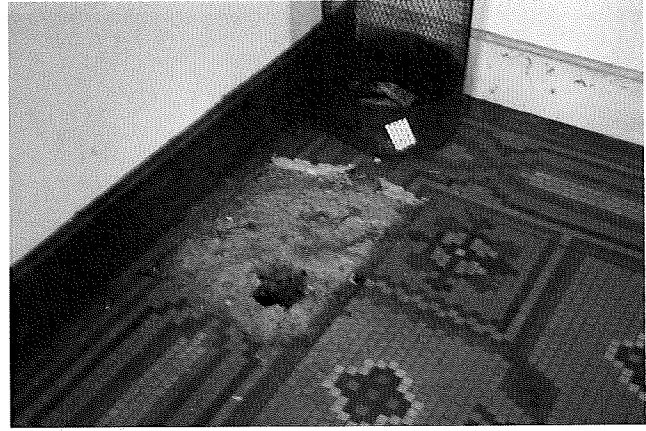
First Floor: View at back of room where the floor has been removed
