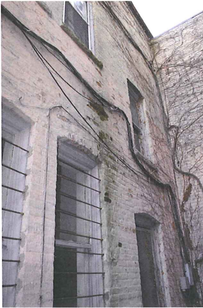
Exterior: View of the back of building showing eroding brick veneer
