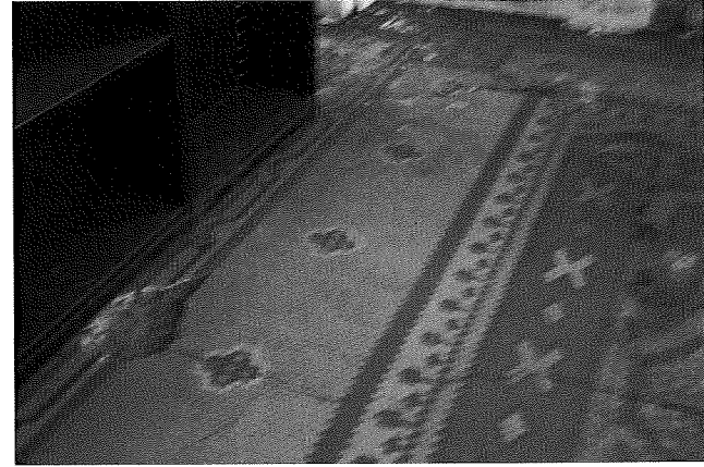
First Floor: View at back of room showing areas where tile floor has been removed
