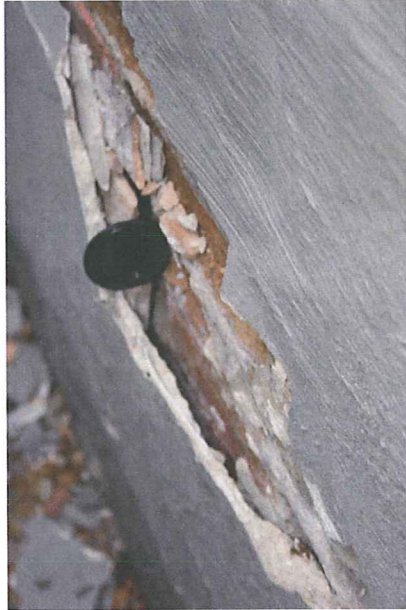
Exterior: View in the alley showing the delamination of the parging system from the brick veneer
