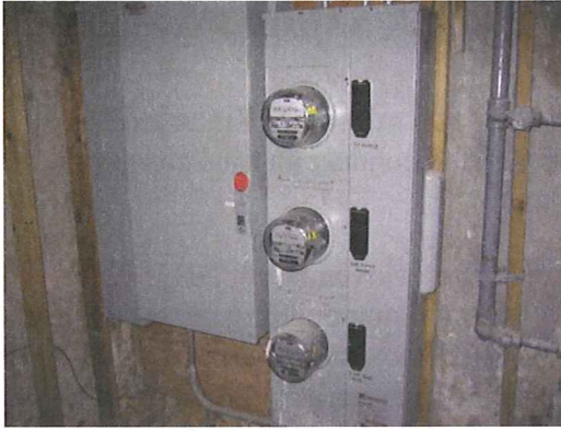
Electrical service in the basement.
