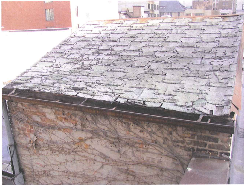
Figure 13. The penthouse roof is covered with asphalt shingles in deteriorated condition.
