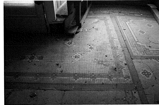
First Floor: View at entry off Mifflin Street showing three flooring surfaces. 1) Original 3/4" square tiles 2) 1" square tiles at entry 3) composite flooring at window
