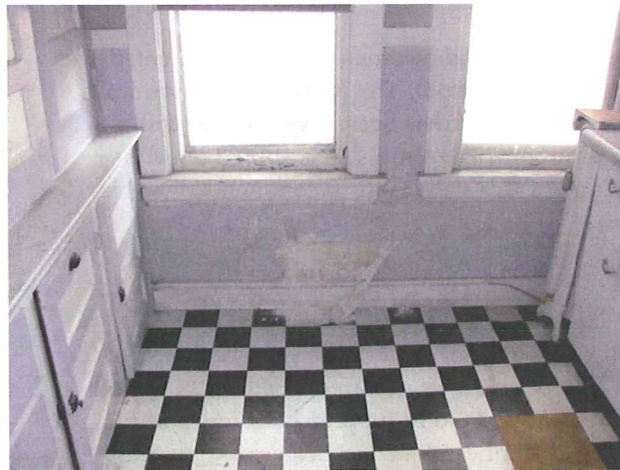
Figure 18. Plaster damage at the rear wall at the second floor of the building.
