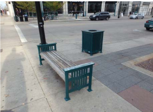
Martin Luther King Jr. and East Main sidewalk (paint chipping, wood fading)
