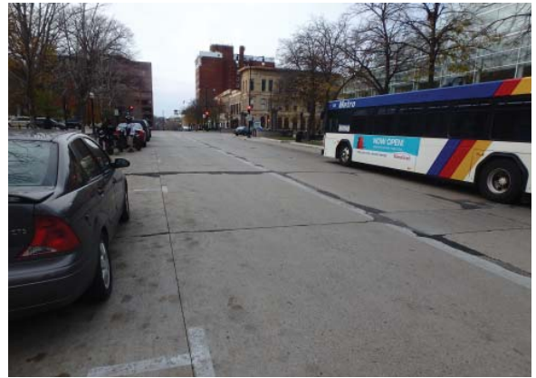
Pinckney looking to East Washington (cracks, patching, fading)
