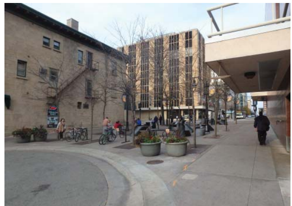
Mifflin plaza (some cracking in cul-de-sac, overall good condition)
