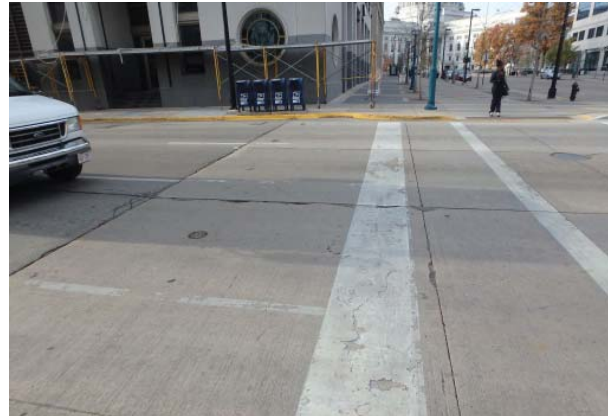
Doty at Martin Luther King Jr. looking north (cracks, patching, chipped paint)
