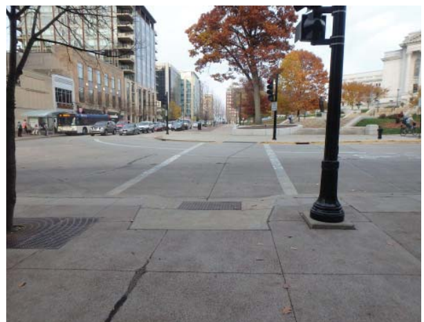
Carroll at Mifflin looking north (cracks, patching)
