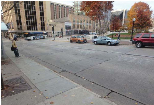
Carroll at West Washington looking West (cracks, patching, fading)
