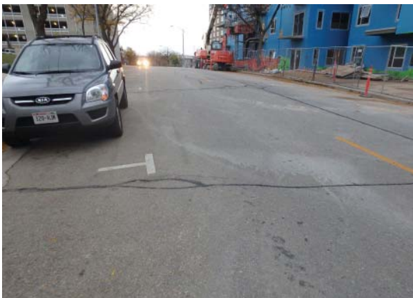
Henry at Main looking east (patching, staining )
