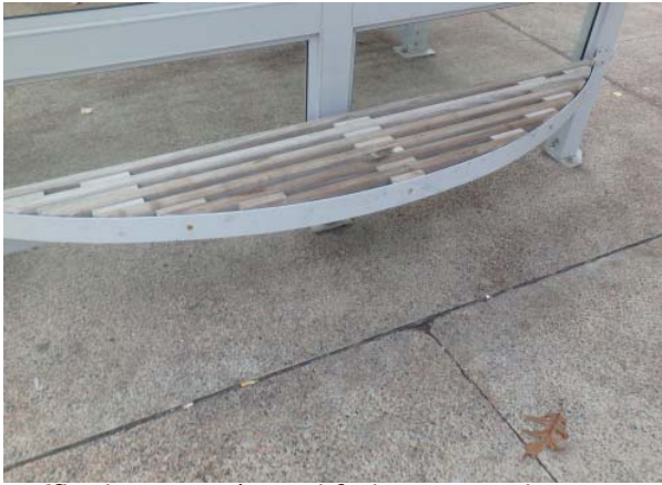
Mifflin bus stop (wood fading, rusted screws, some cracks in sidewalk)
