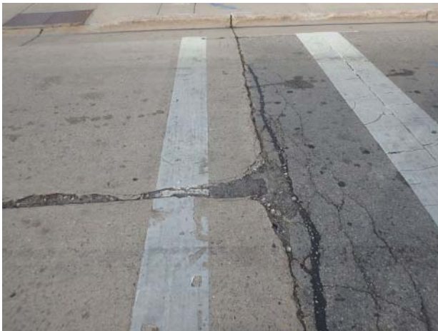
Carroll at Hamilton (patching, cracks, stains)
