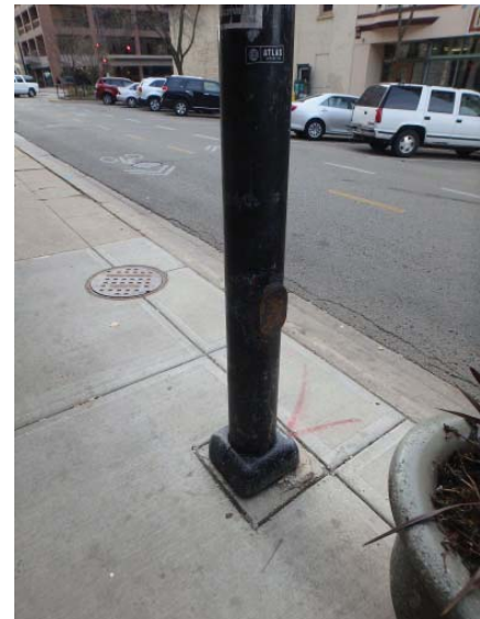
East Mifflin light pole (rust near bottom)
