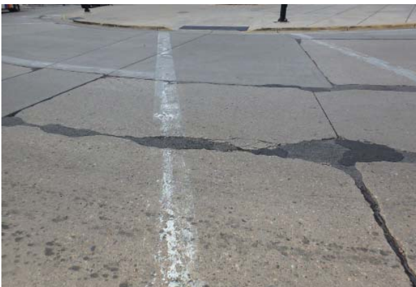
Doty at Carroll (patching, fading, cracks)
