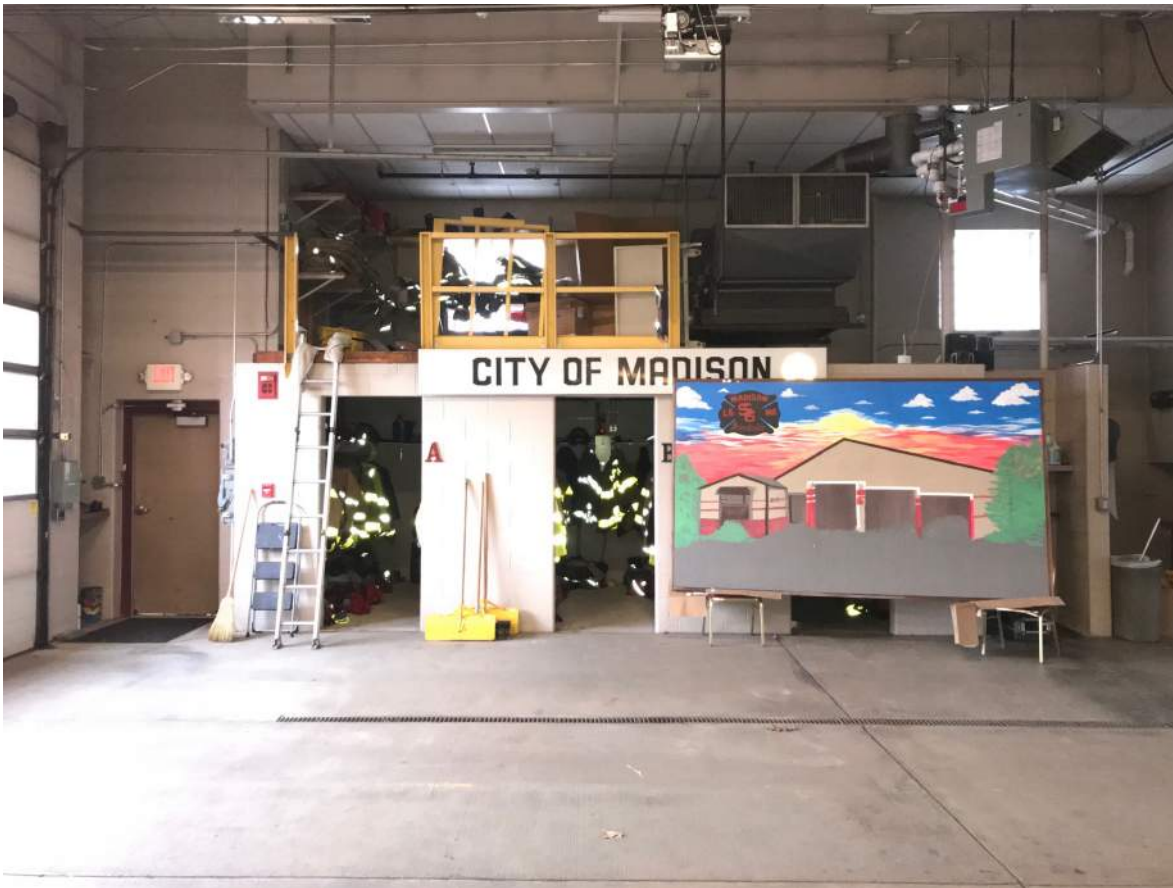
Fire Station 6 interior of apparatus bay facing west. Exterior wall to be removed to accommodate proposed addition.
