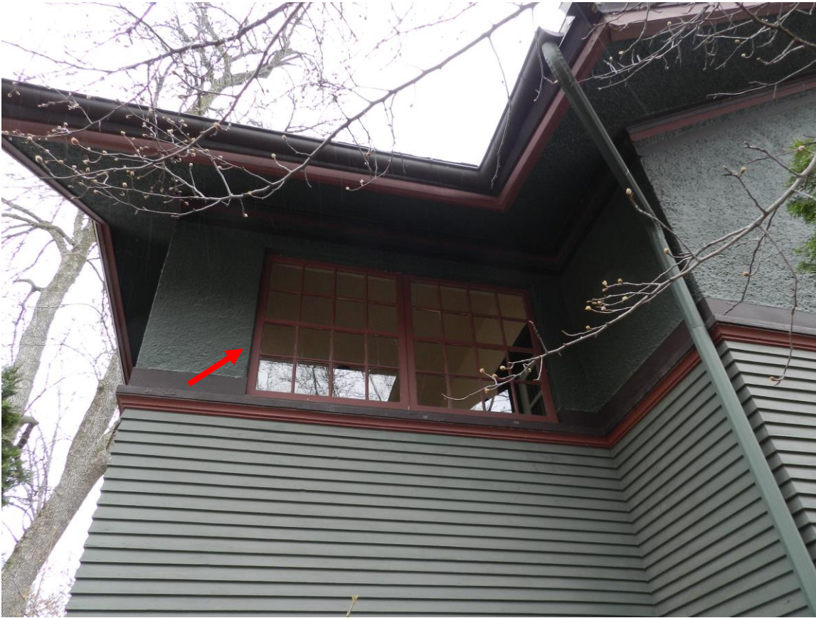
West side upper porch windows to be replaced
