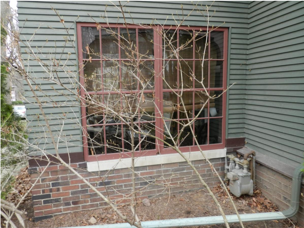
West side lower porch windows (These windows are not being replaced and will remain as is)
