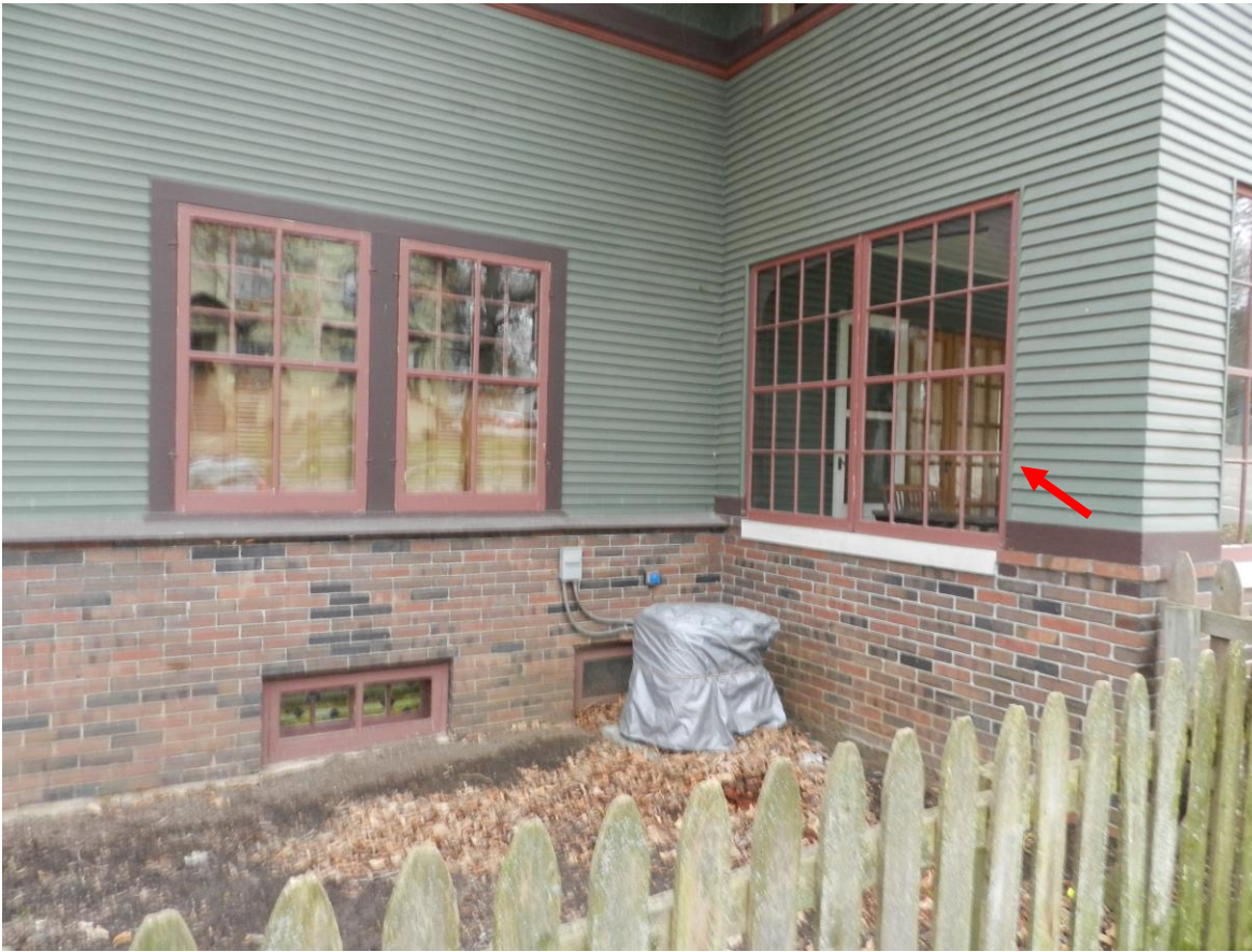
East side lower porch windows (These windows are not being replaced and will remain as is)
