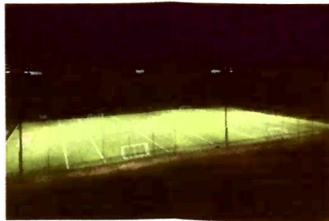
An example of Edgewood's proposed lighting system installed at Clemson Field
