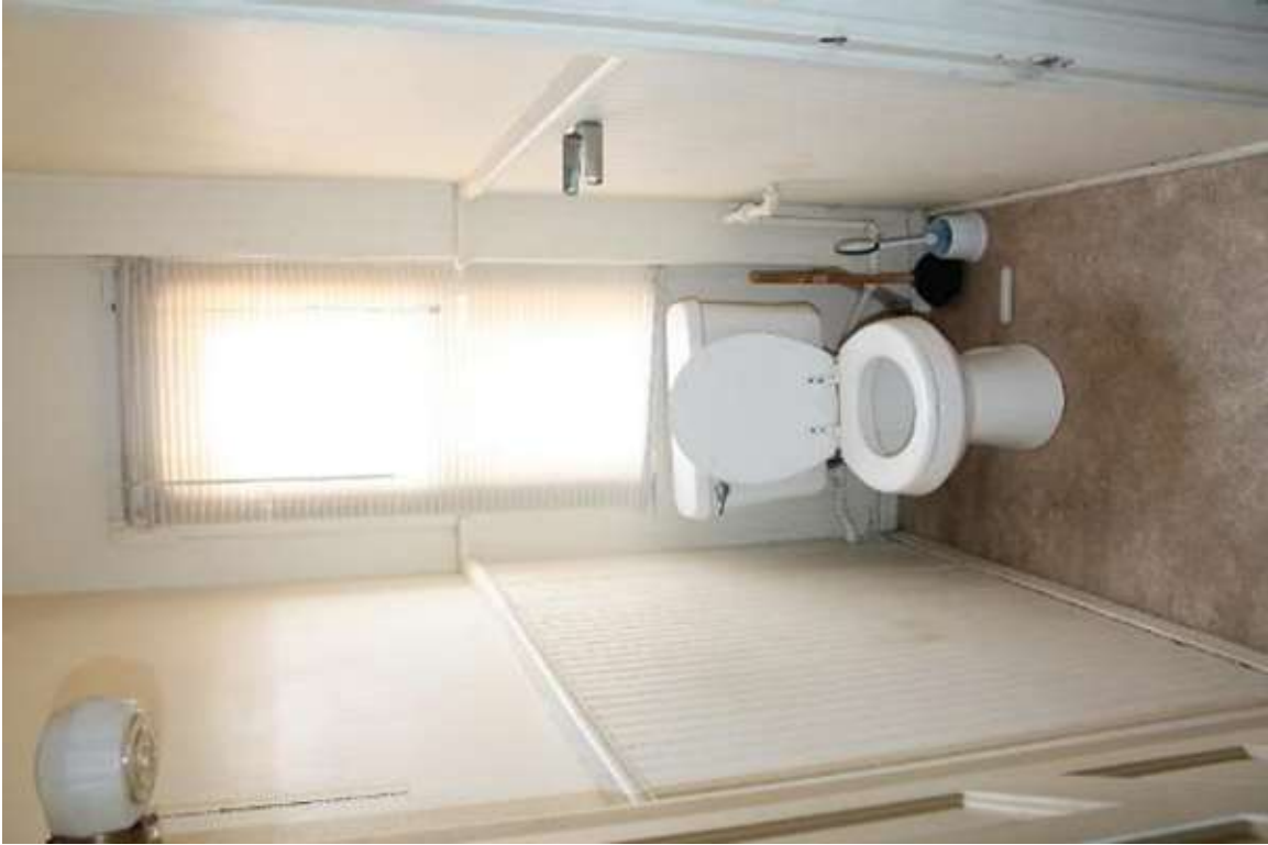
Photo 37: 9 North Hancock Street, Interior, second floor toilet
