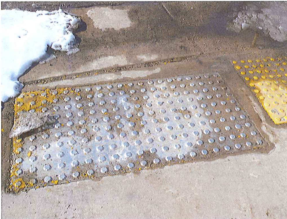
Stainless steel panel with complete surface failure
