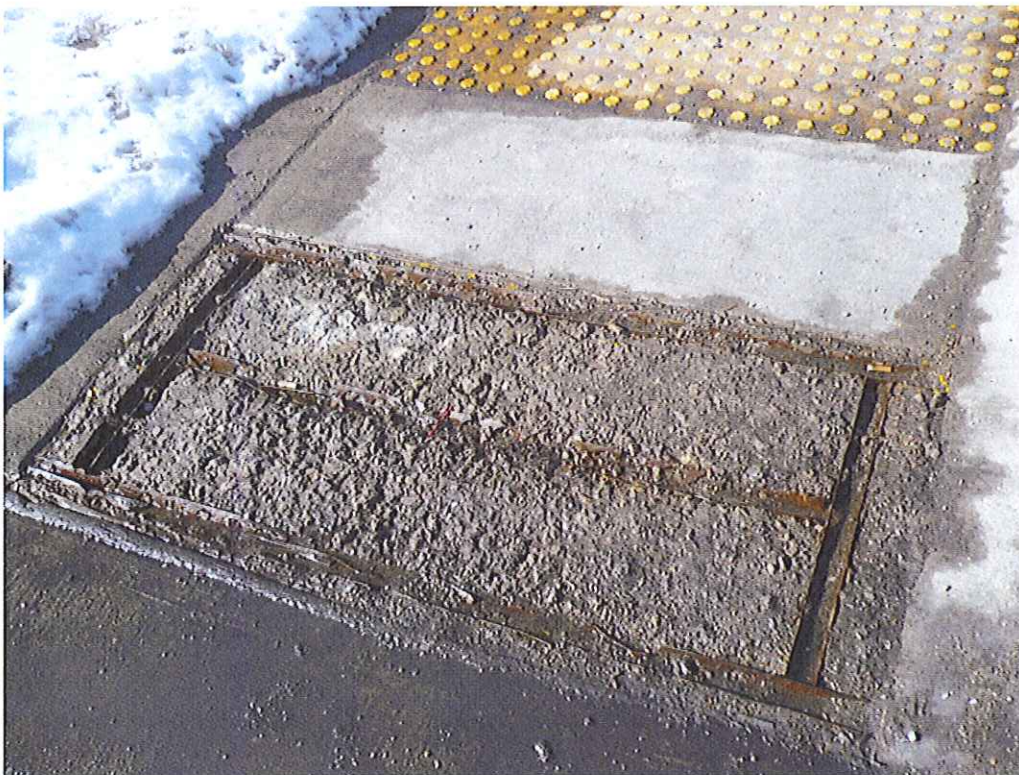
Stainless steel panel torn from concrete surface after edge pulled up at 2 nd Street and E. Washington Ave.
