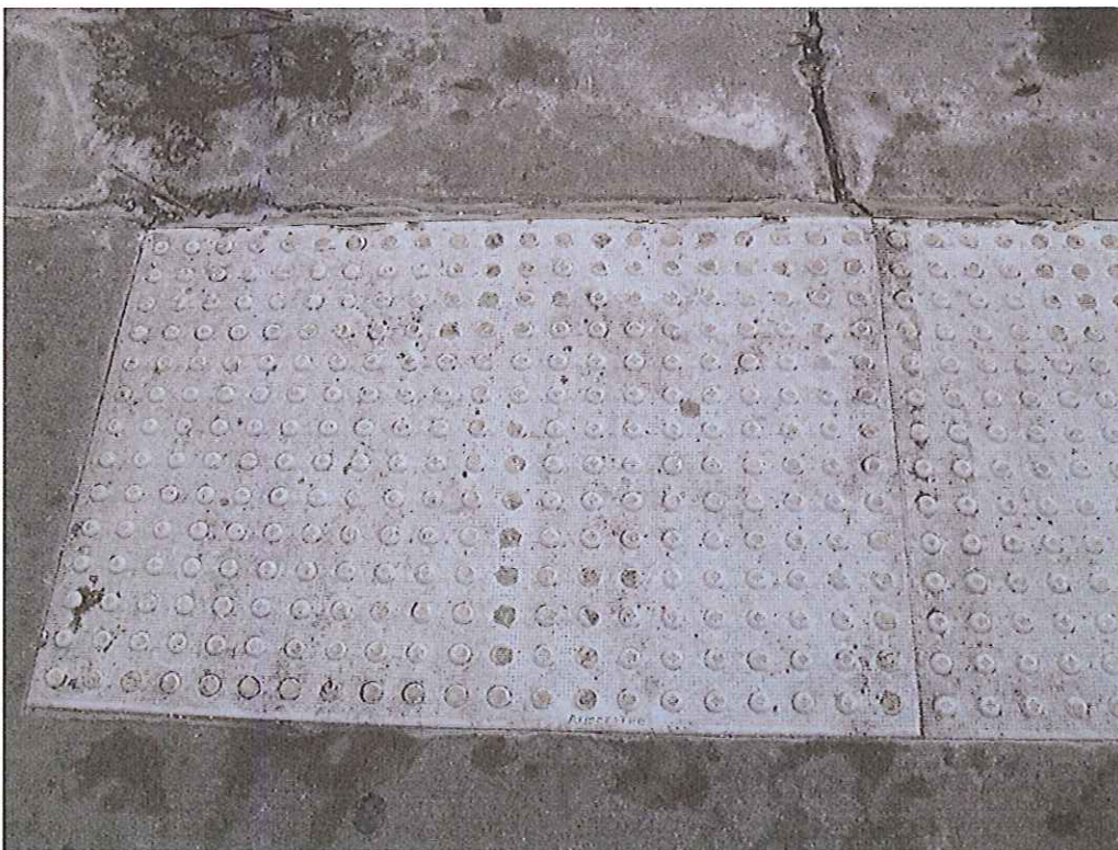
Composite Panel – Domes removed from wear and/or snow removal operations
