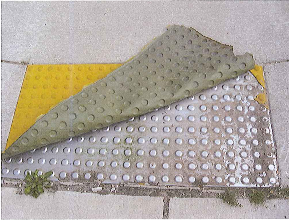
Stainless steel plate with peeling surface
