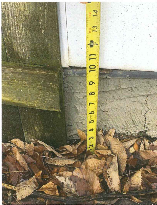
North West corner, approx 9.25" from grade (different segment of foundation, addition concrete)
