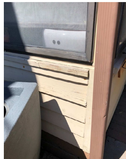
ROTTEN SILLS LEFT SIDE OF "BOX"
