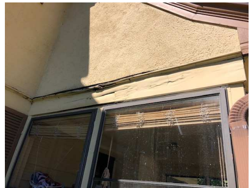
ROTTEN BEAM AT LEFT SIDE OF "BOX"
