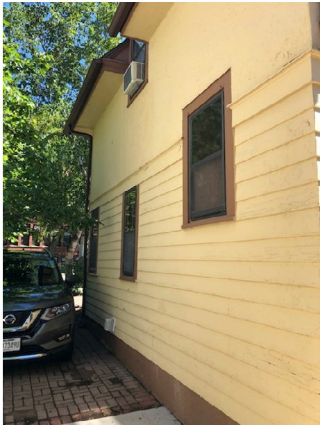
BLOCKED UP KITCHEN WINDOW
