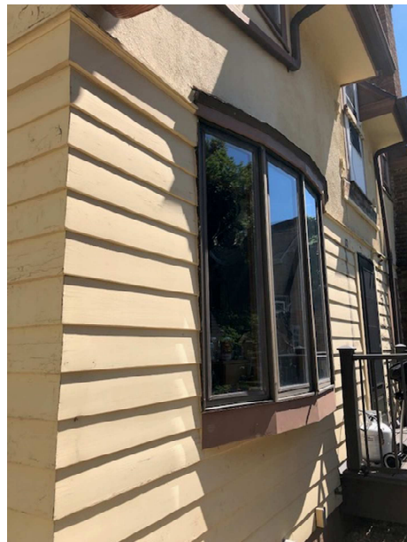
BAY WINDOW TO BE REPLACED
