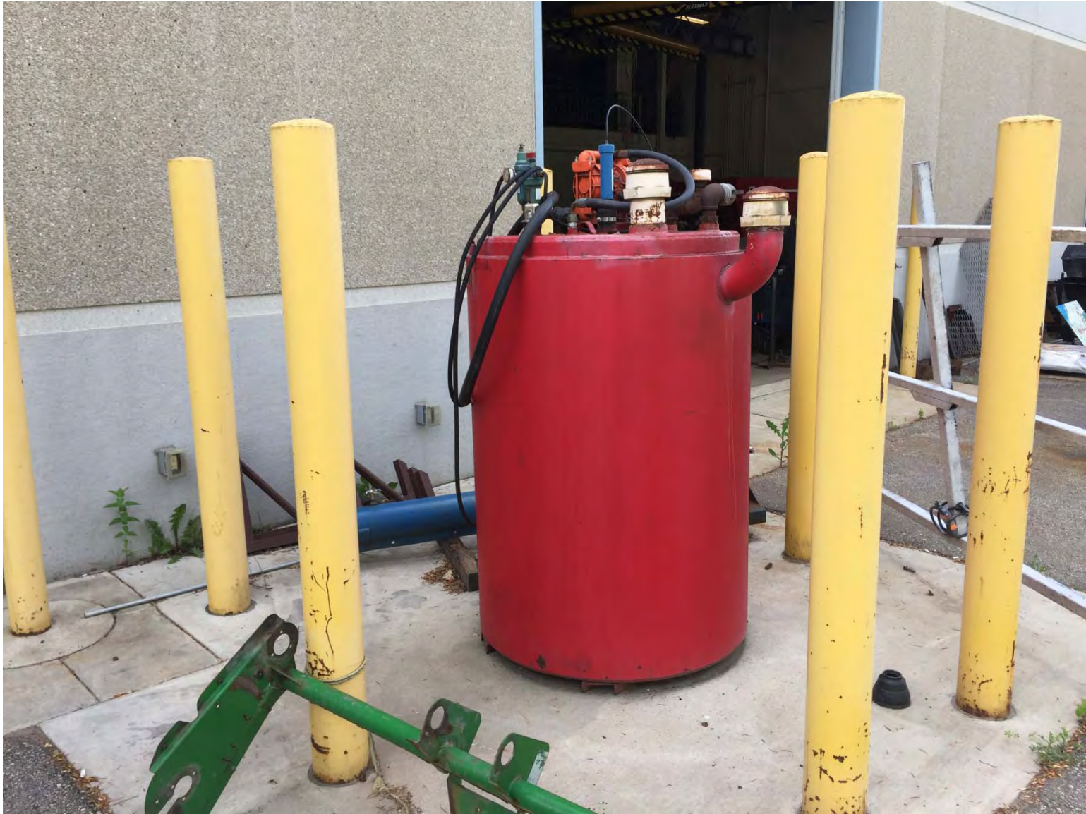
Parks Goodman Yard M-15 : Outdoor Waste Oil Storage
