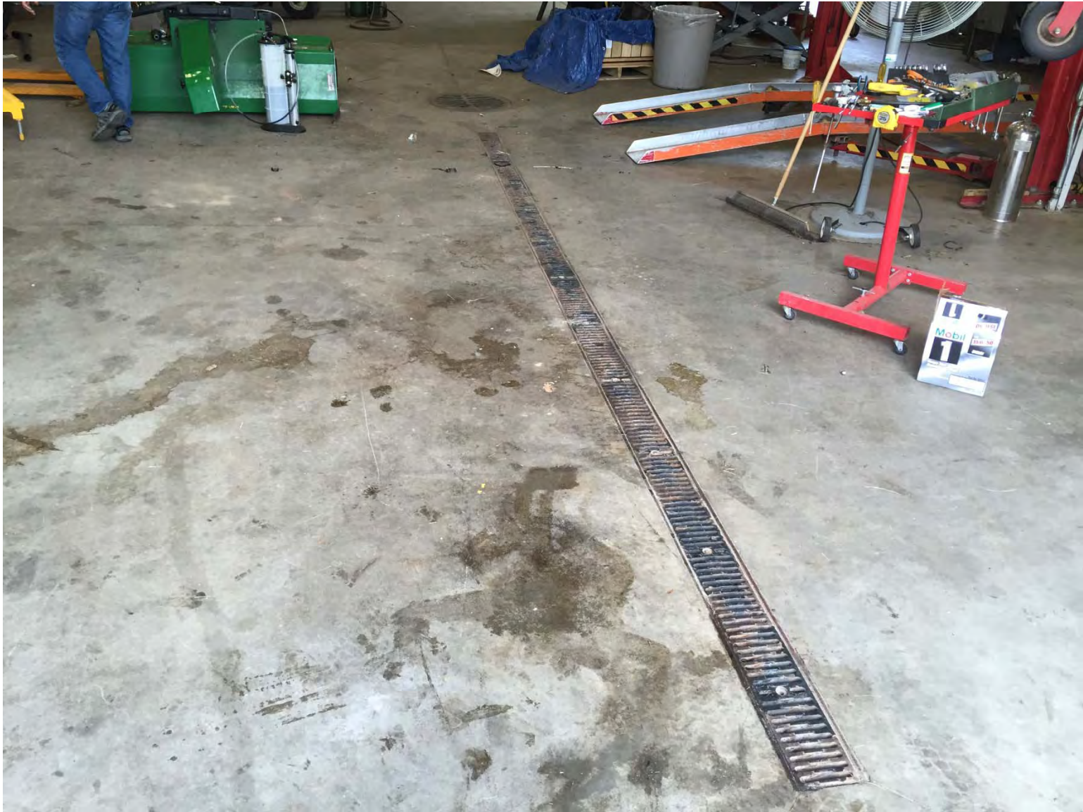
Parks Goodman Yard B2-43: Vehicle Maintenance, Metalworking Shop Trench Drain
