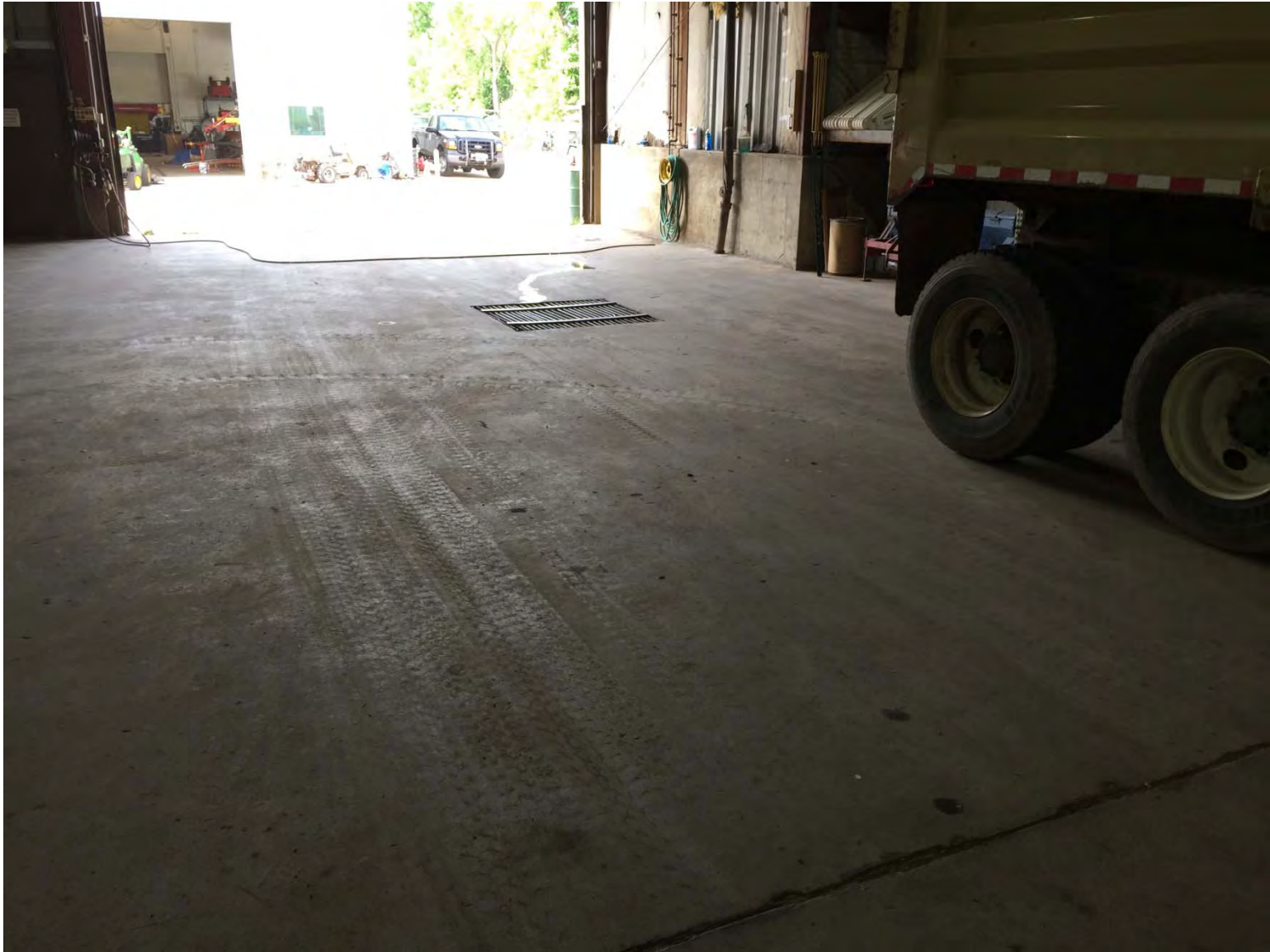
Parks Goodman Yard B1-4: Floor Drain
