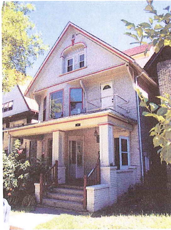
View of the front 19 N. Webster. The porch has several deterioration issues.
