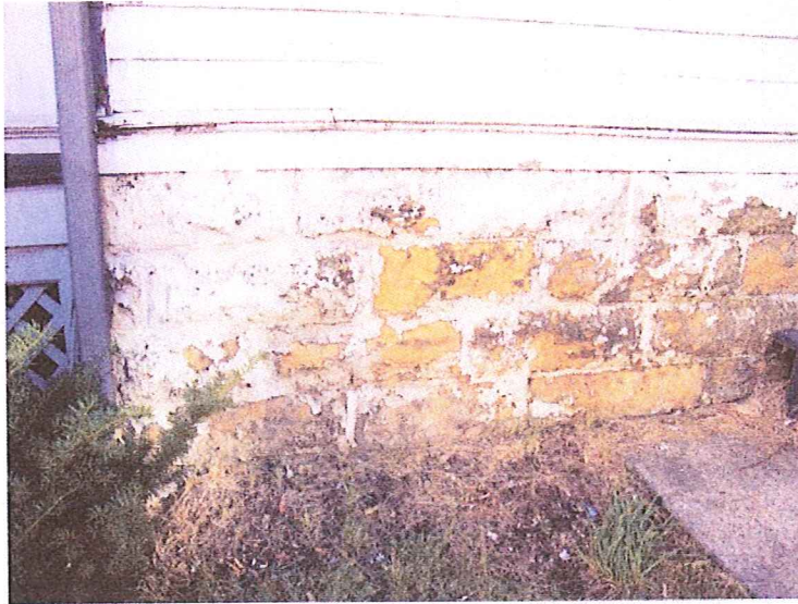
Image of 201 E. Mifflin St. showing the deterioration of the stone masonry foundations walls
