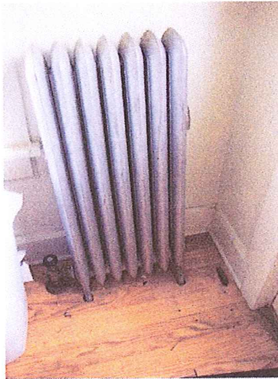
Typical hot water radiator. 17 N. Webster St first floor apartment.
