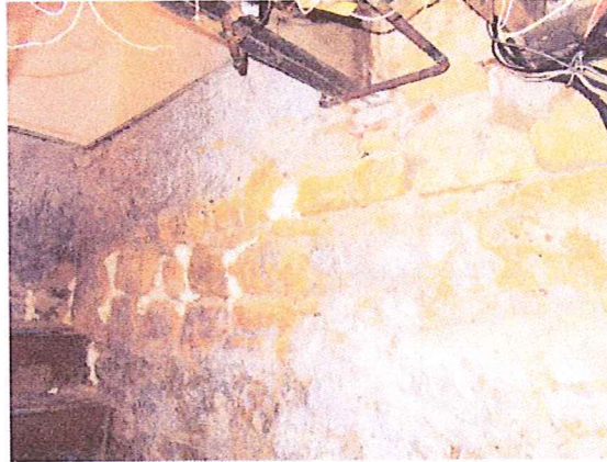
Image showing deteriorated stone foundations and spray insulation filler at 19 N. Webster St.
