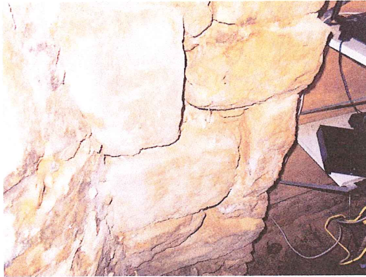
Image showing significant deterioration of mortar in foundation walls 17 N. Webster St.
