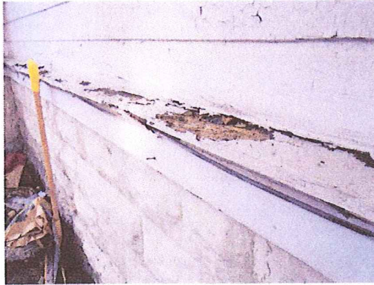
Image showing water infiltration and location of possible damage to framing at the water table trim. East side of 201 E. Mifflin St.
