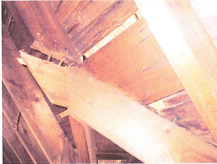
Image showing damaged roof framing at dormer framing. 17 N. Webster St.
