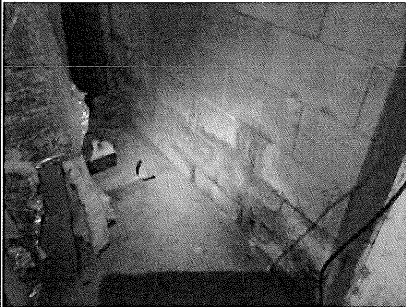
- Basement walls have Efflorescence present. Indicating water is present on exterior of wall pushing through. Recommend further evaluation and maintaining a positive grade away from foundation.
