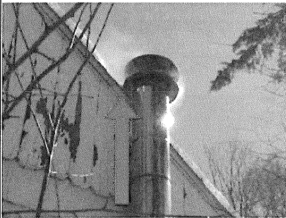
- Metal furnace chimney is not high enough over roof. Recommend repair.
