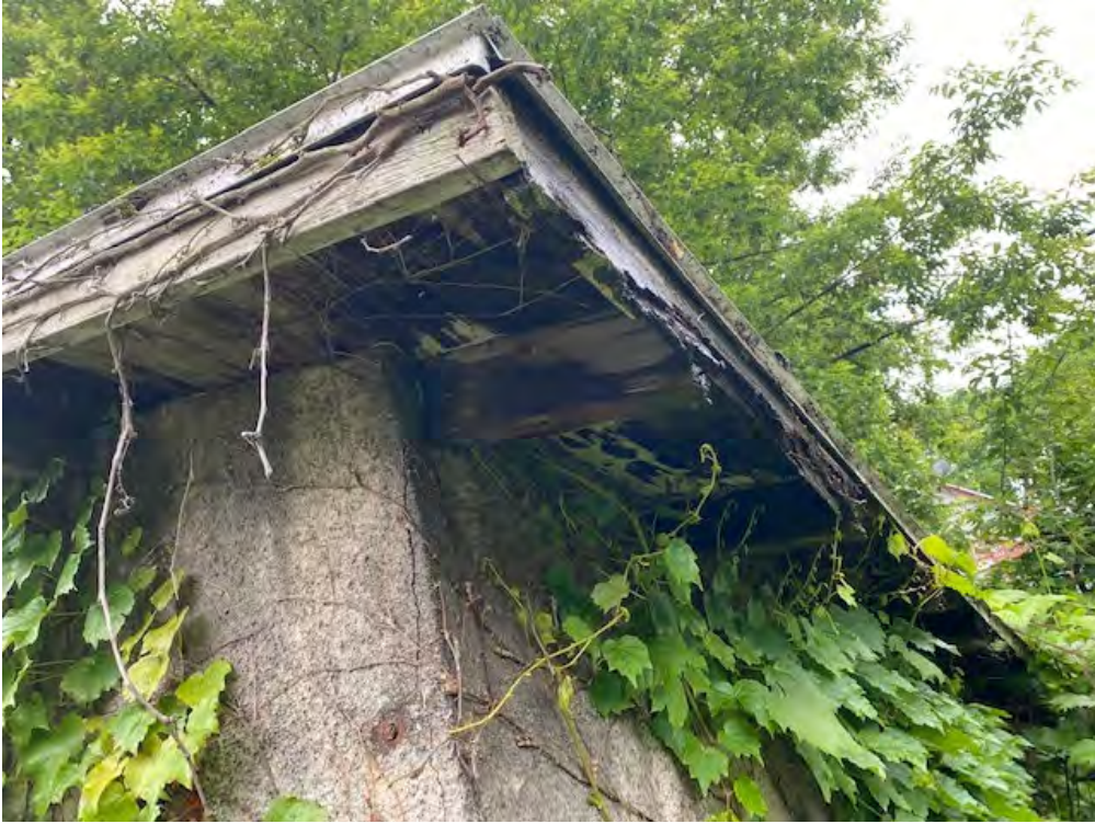
Rafter ends deteriorated
