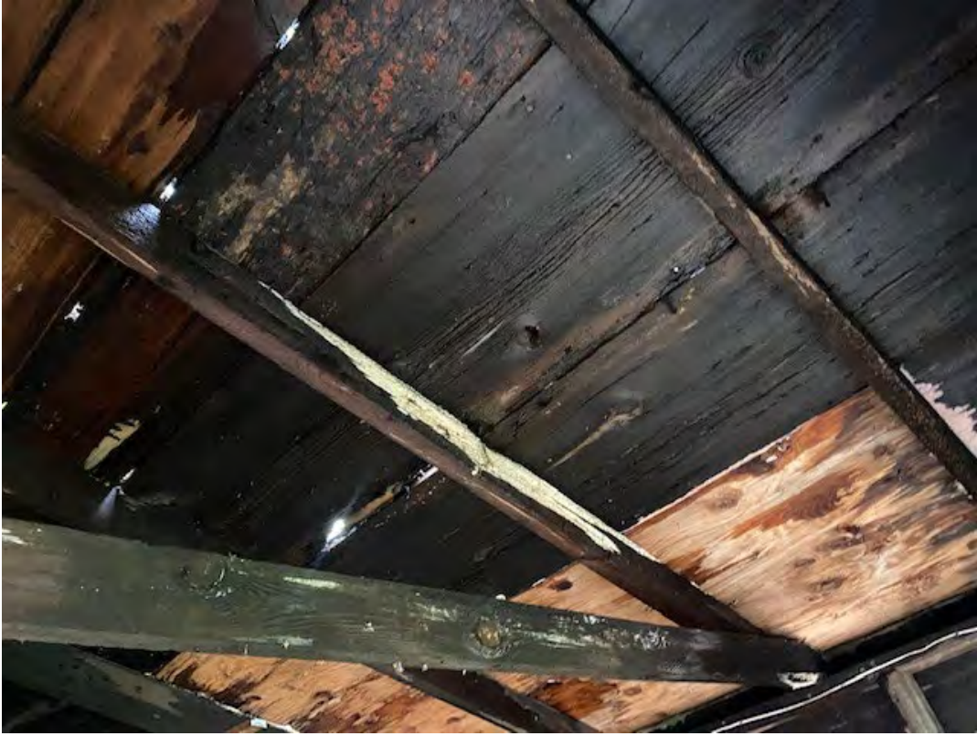
Holes in roof
