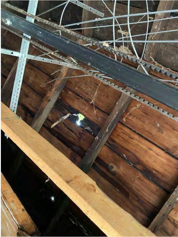
Holes in Roof
