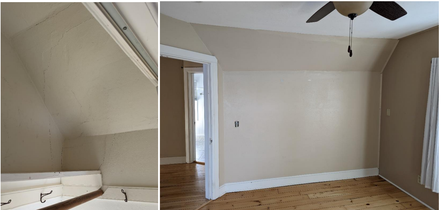
Images of upper level plaster cracking and roof structure deformation.
