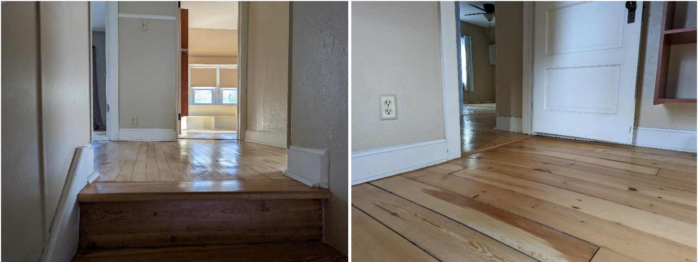
Images of upper level canted floors and uneven structure settling.
