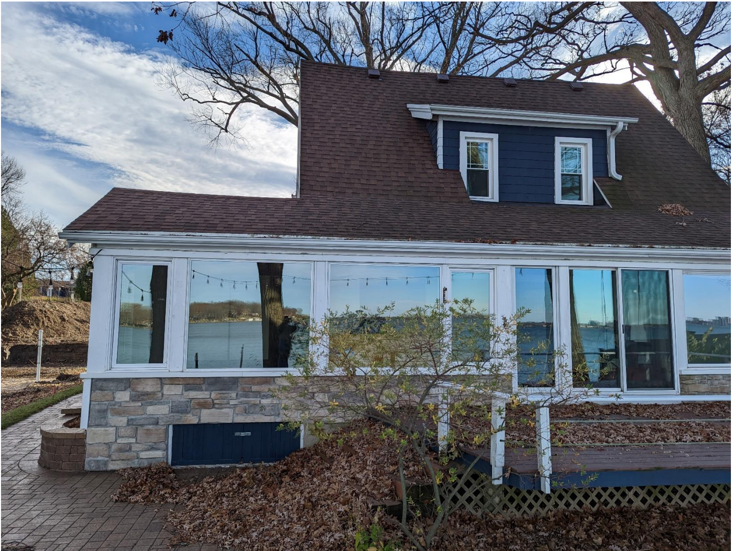
Lake Facing Building Elevation – Note sagging roofline at lower and upper roof ridges.
