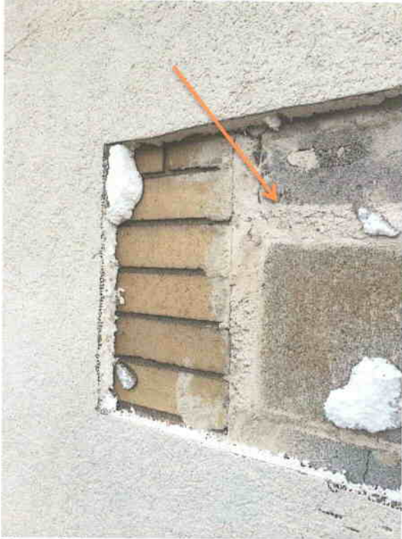
View of the concrete block infill used where original windows and doors were removed. August 20, 2015.
