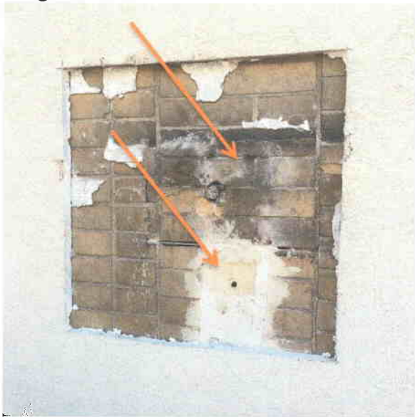
Image of brick area where original applied decorative trim was removed and void infilled with mortar. October 1, 2015
