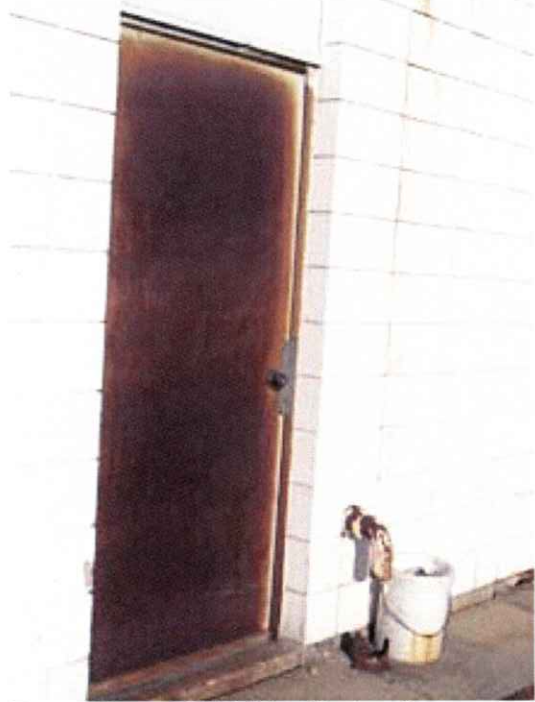
Rusted Door-854 E. Washington Avenue
