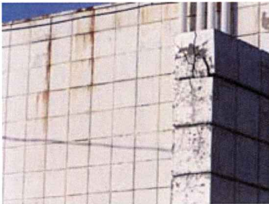
Broken & Deteriorating Block 854 E. Washington Avenue
