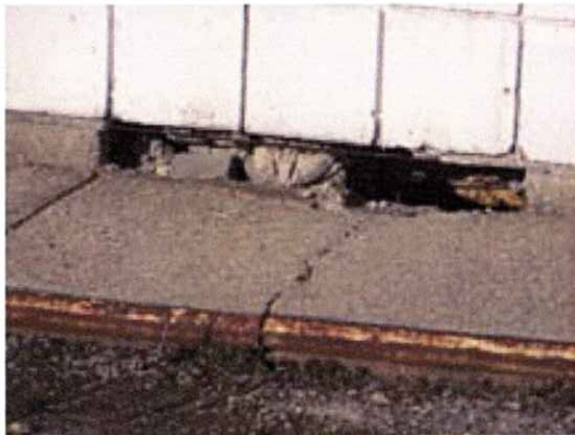
Broken Foundation & Sidewalk 854 E. Washington Avenue
