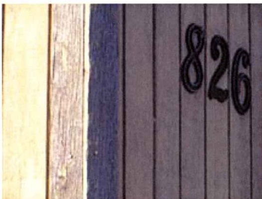
Deteriorating Siding 826 E. Washington Avenue
