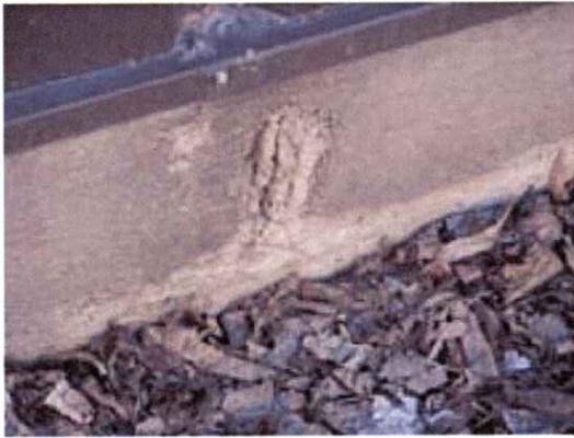
Deteriorating Foundation-837 E Mifflin Street
