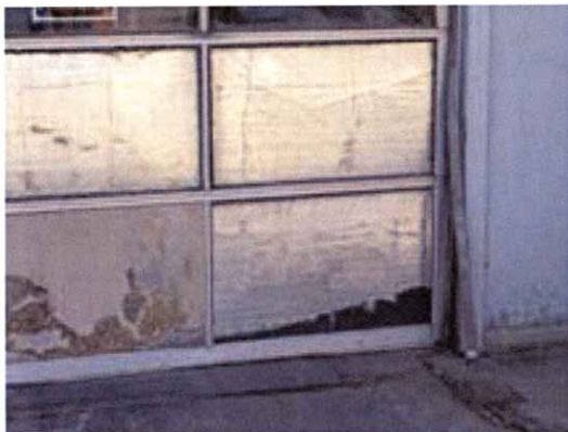
Cracked Glass – Loose Door Frame- 854 E. Washington Avenue
