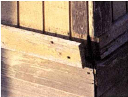
Loose Trim & Deteriorating Siding 826 E. Washington Avenue
