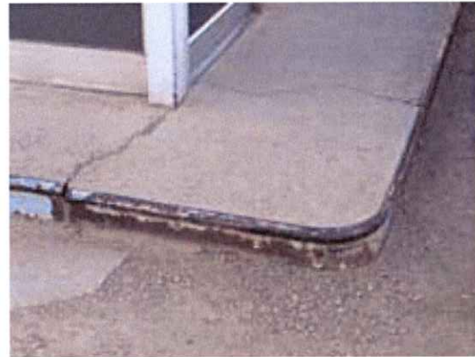
Cracked Sidewalk 854 E. Washington Avenue
