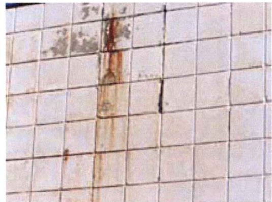
Deteriorating Block-854 E. Washington Ave
