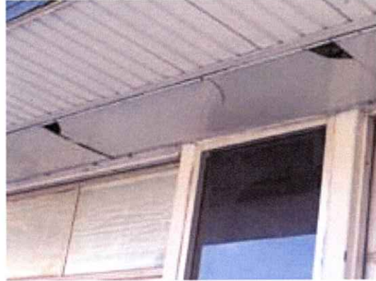
Broken Soffit – 854 E. Washington Ave
