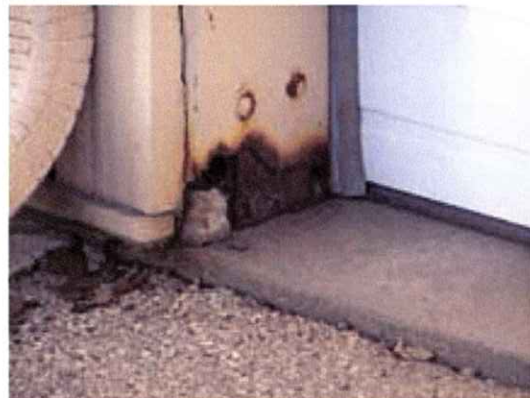
Rotted Door Frame – 835 East Mifflin Street
