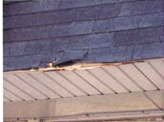
Deteriorating Fascia 854 E. Washington Ave
