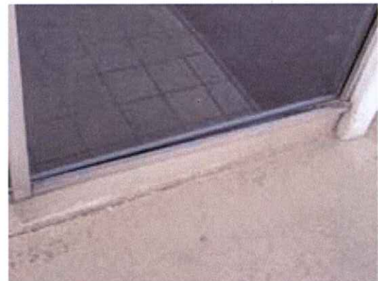
Loose Window Trim 854 E. Washington Avenue
