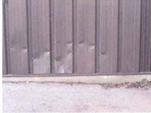
Dented Siding – 837 E. Mifflin Street
