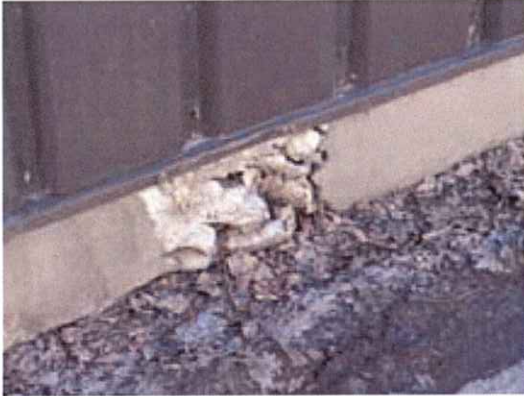
Broken Foundation – 837 E. Mifflin Street
