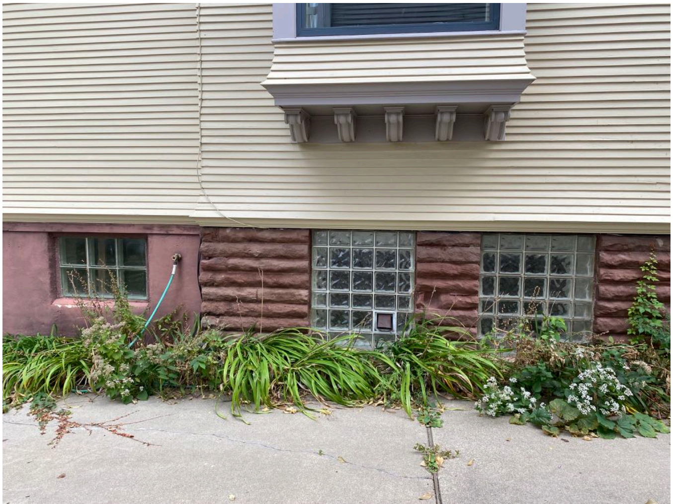
Photo of Existing Dryer Vent on East Facade (Item 4) and Existing Glass Block Windows (Item 11)
