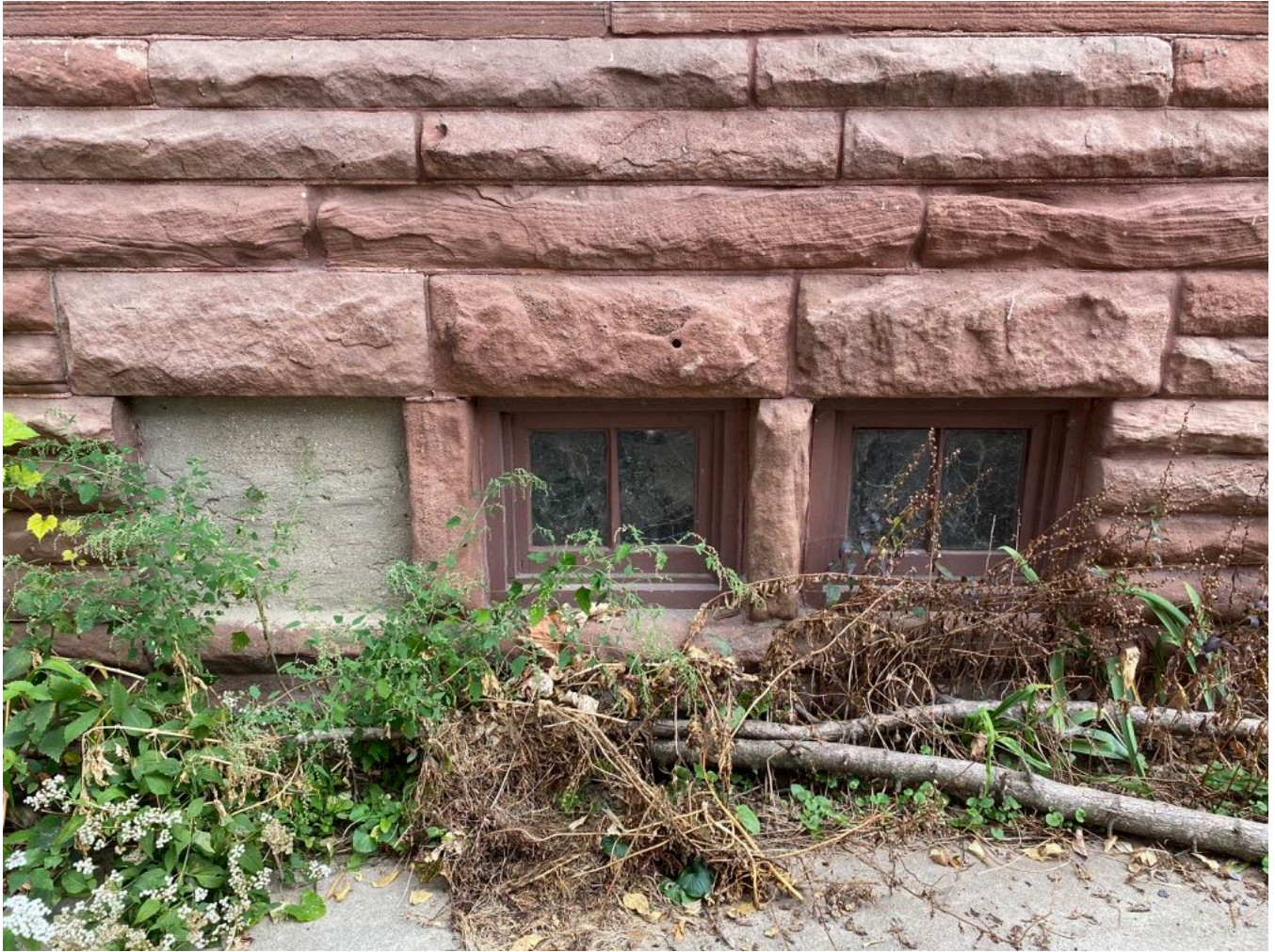
Photo of Existing Missing Window (Item 9)
