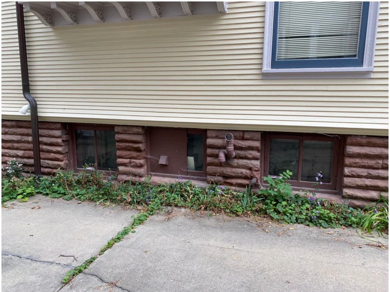
Photo of Existing Utility Venting on West Facade (Item 2) and Damaged Window (Item 10)
