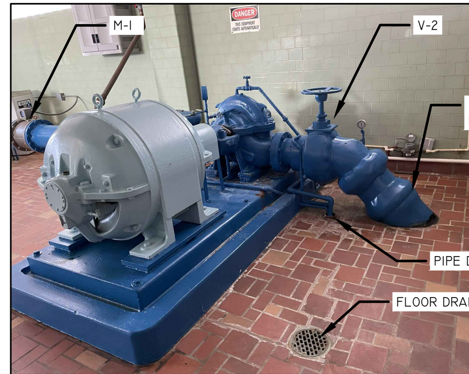
EXISTING PUMP AND MOTOR FACING NORTHWEST
