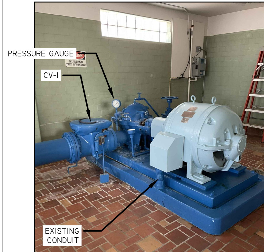
EXISTING PUMP AND MOTOR FACING NORTHEAST CORNER
