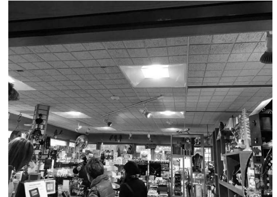
EXTG GIFT SHOP CEILING: EXTG CEILING TILES TO BE REPLACED, GRID TO REMAIN.
