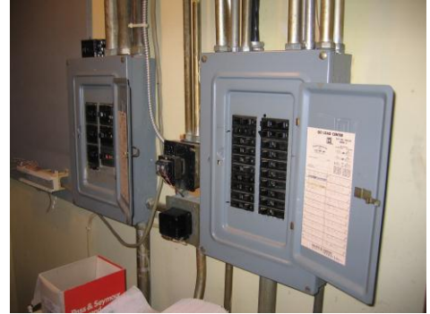
Electrical panels on 2 nd floor.
