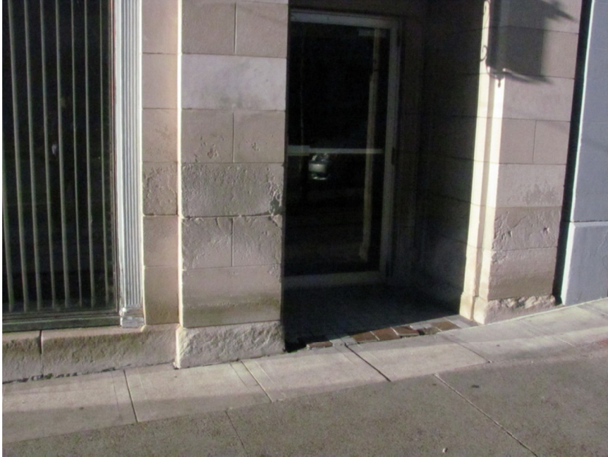
Figure 4. Portions of the limestone masonry near grade exhibit erosion and pitting of the face.
