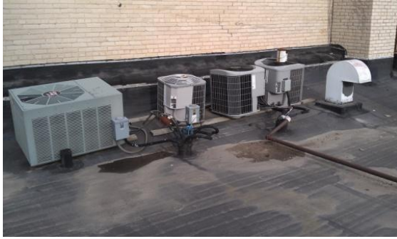
Condensing units serving the furnaces
