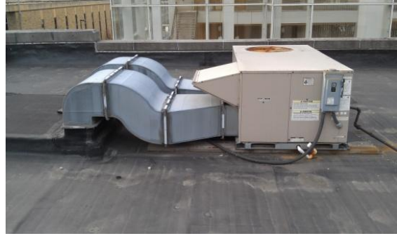
One of two packaged rooftop units
