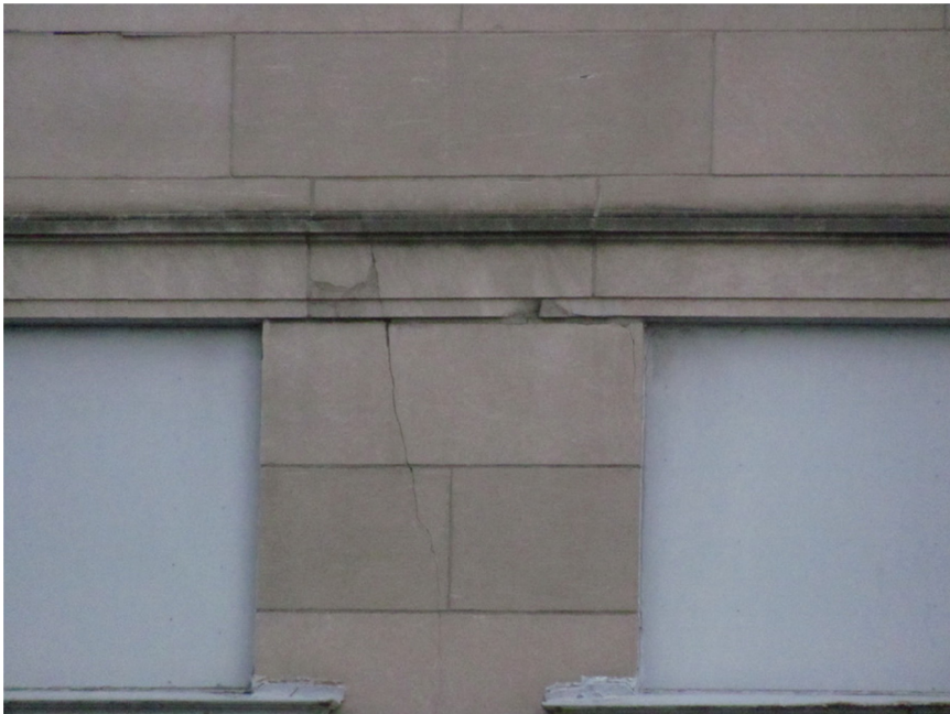
Figure 5. Cracking and spalling of limestone masonry at the head of a first floor window opening.
