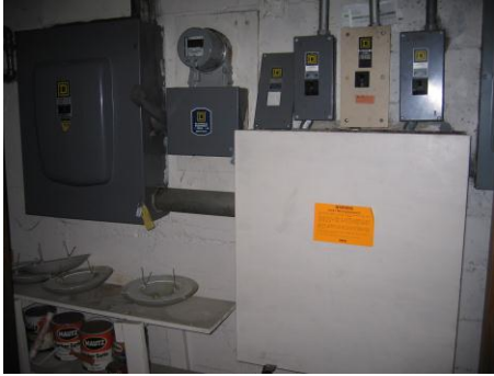
Electrical service in the basement.
