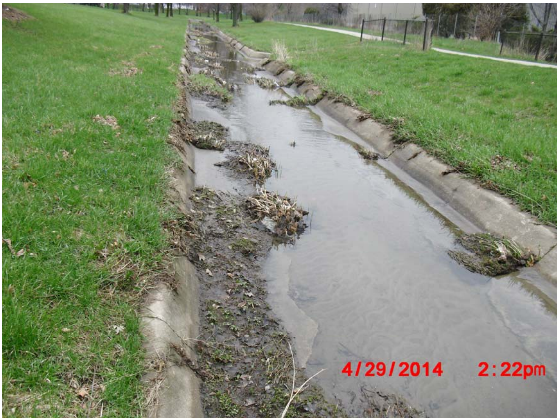
Photograph 3: Existing conditions of the channel. Degraded concrete and sediment deposition are both visible in this photo.
