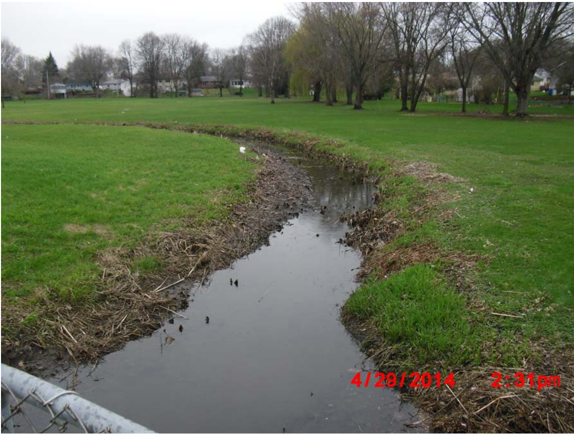
Photograph 4: Existing conditions of the channel. The final 400 feet of the channel are an unlined ditch.
