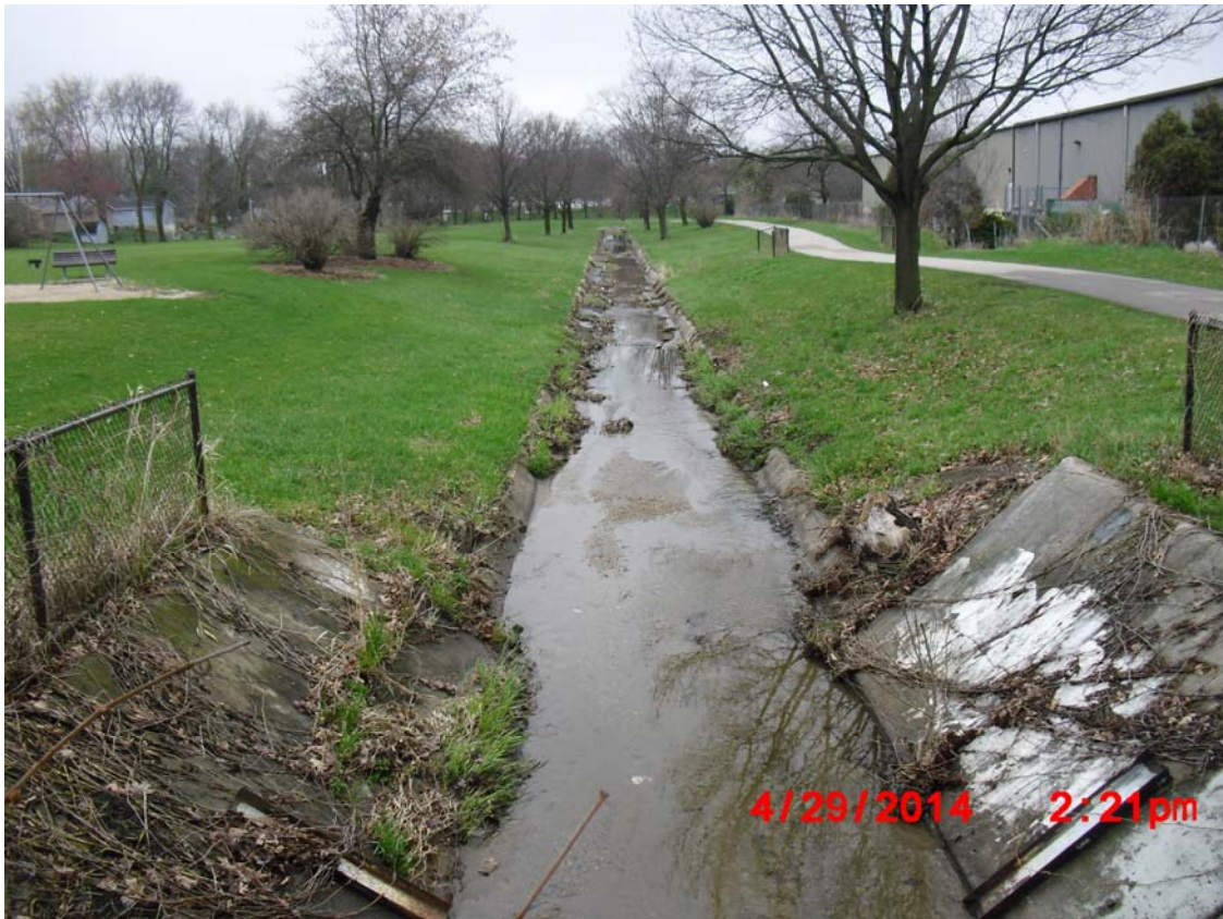
Photograph 2: Existing condition of the channel. This photo was taken from the furthest upstream point.
