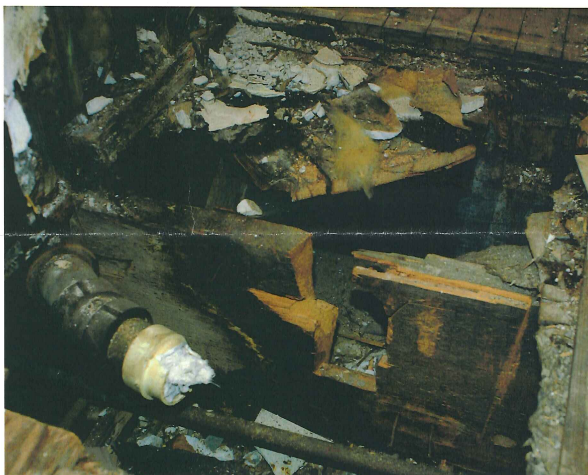
632 HOWARD PLACE EXISTING CONDITION UNDERNEATH THE FLOOR - NOTE SEVERE DETERIORATION OF THE FLOOR SHEATHING AND COMPROMISED FLOOR STRUCTURAL FRAMING DUE TO PREVIOUS MECHANICAL, ELECTRICAL AND PLUMBING INSTALLATION AND REPAIR - THIS CONDITION IS NOTICEABLE AND LIKELY PRESENT IN ALL UNITS - THE SOLUTION TO THIS CONDITION WOULD LIKELY REQUIRE A TOTAL FOUNDATION UP REBUILD OF THE ENTIRE STRUCTURE
