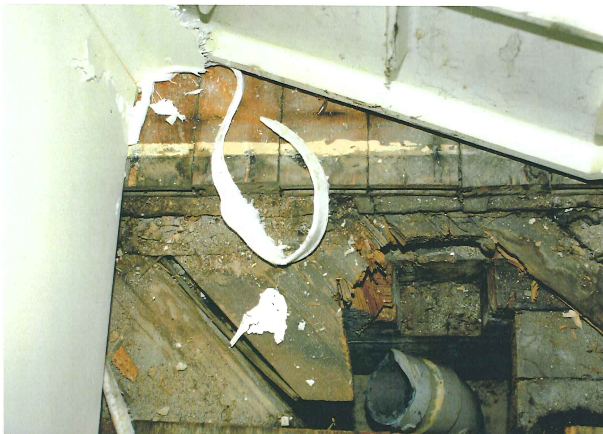
632 HOWARD PLACE TYPICAL CONDITION AT THE EXISTING INTERIOR FLOOR STRUCTURE - SEVERE DAMAGE TO THE FRAMING AND FLOOR SHEATHING - LAKE TOWNE APARTMENTS HAS IMPROVED THE UNITS WERE NECESSARY AND PRACTICAL
