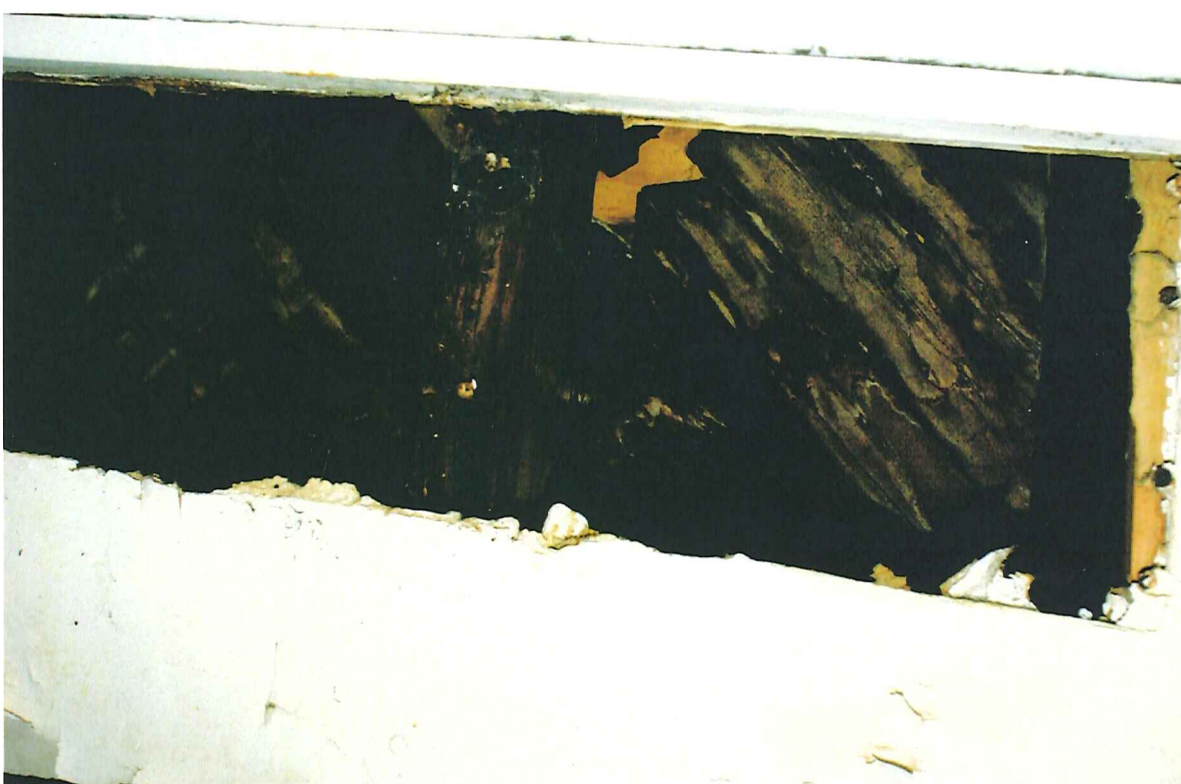
632 HOWARD PLACE IMAGE TAKEN OF UNDERSIDE OF FLOOR FRAMING AND FLOOR DECKING SHOWING SEVERE AND PERVASIVE WATER DAMAGE - THIS CONDITION IS NOTICEABLE IN EACH UNIT AND IS LIKELY PERVASIVE THROUGHOUT THE ENTIRE BUILDING
