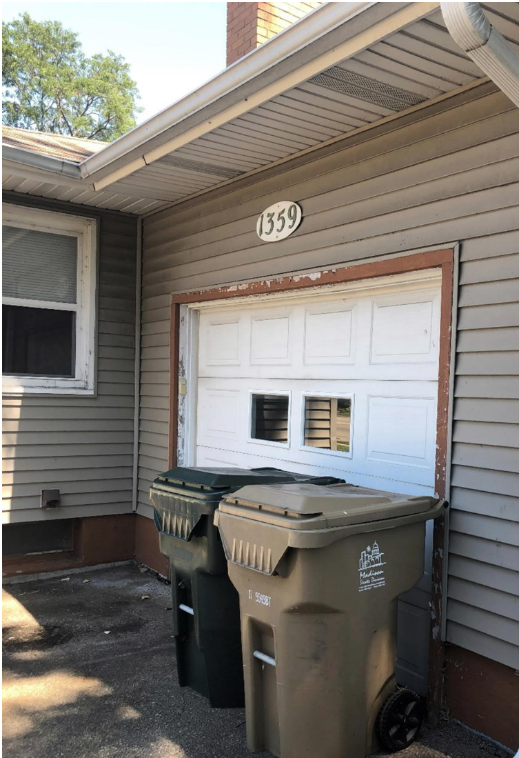
Garage Door - frame not plumb due to structure settlement
