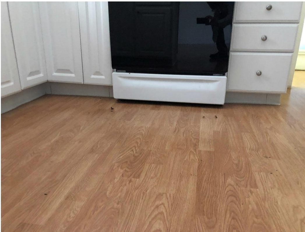
Kitchen floor sloping to left in photo
