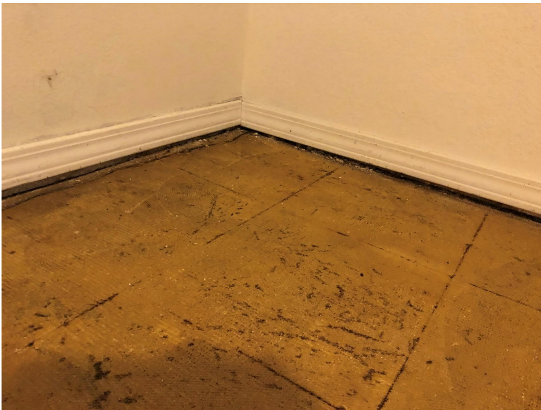
Basement floor/wall joint - note floor settlement
