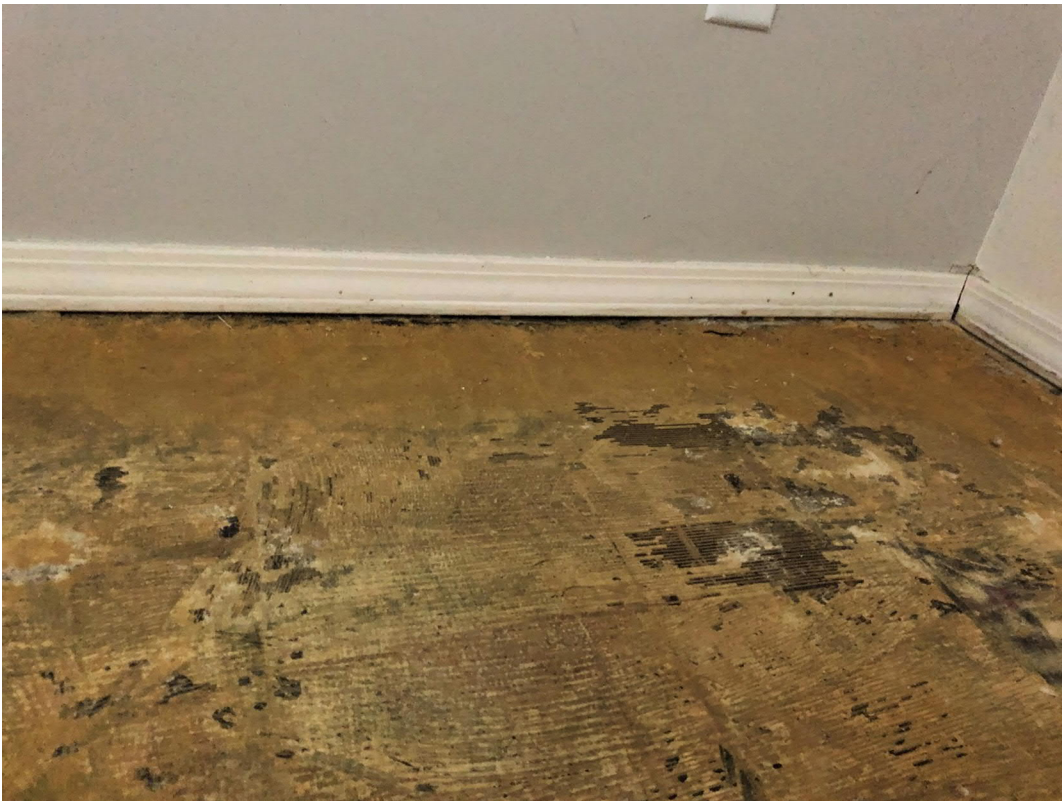
Basement floor/wall joint - note floor settlement
