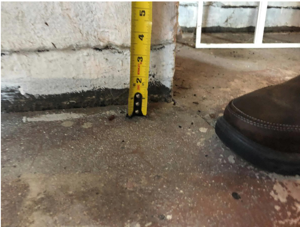
Garage floor - settlement about 3-1/2"
