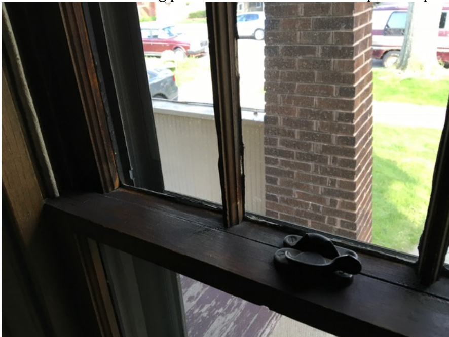
Inside window showing previous unsuccessful attempts at replacing caulking
