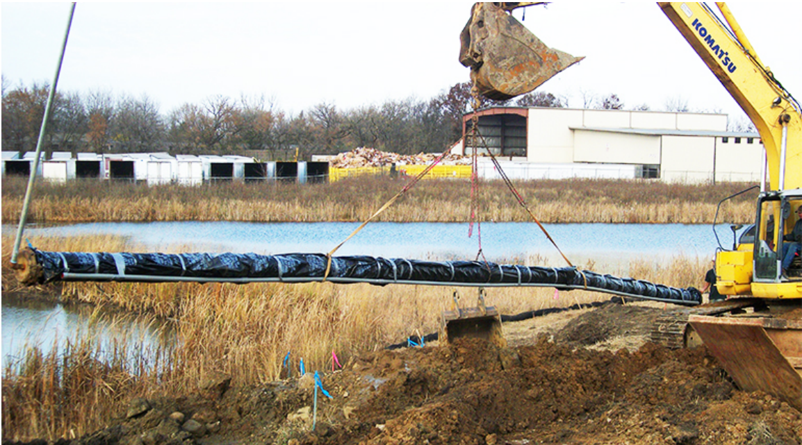
A SECTION OF THE CANNONBALL WATER PIPELINE IS INSTALLED IN SOUTH MADISON, FALL 2019
