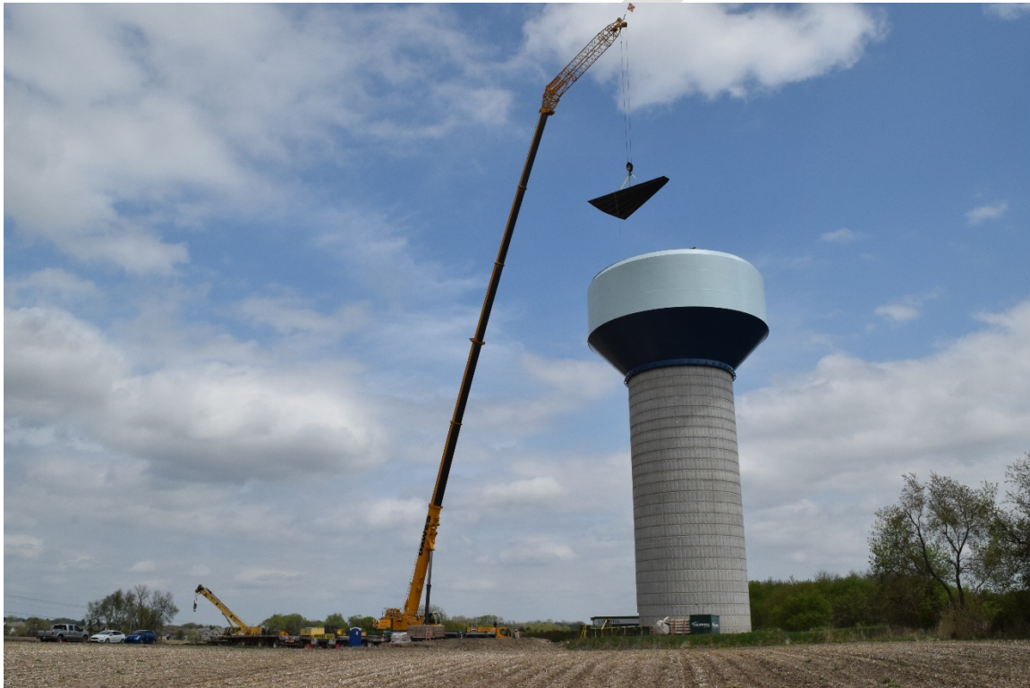
A CRANE LIFTS A SECTION OF THE STEEL ROOF INTO PLACE AT THE TOP OF BLACKHAWK WATER TOWER.
